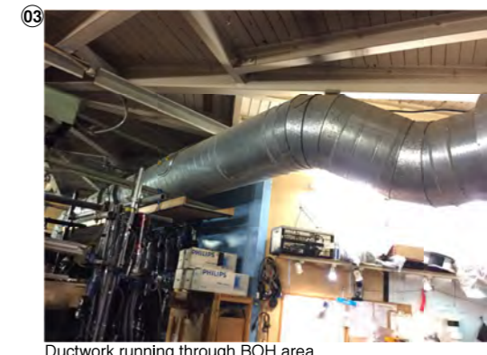
Ductwork running through BOH area
