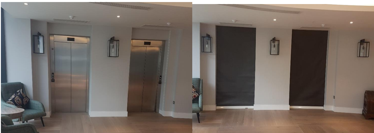
Figure 11 — Lift Lobby protected by fire curtains (left - open and right- deployed)
