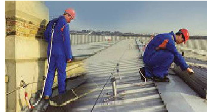
Mansafe cable and lanyard system
