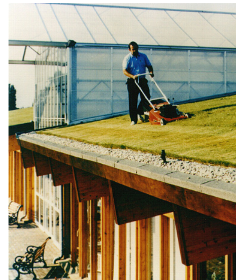
Inappropriate design & access
