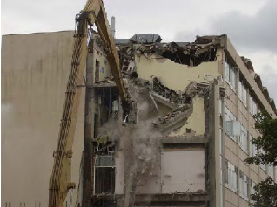
Dust Creation from Demolition
