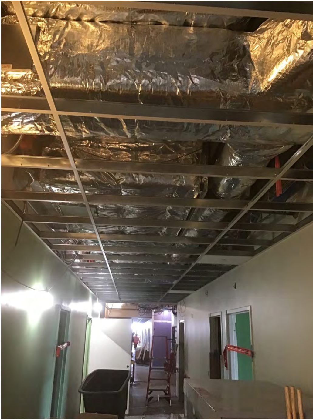
Advancespan™ installed in corridor at Kindred/UC Davis Sacramento.
