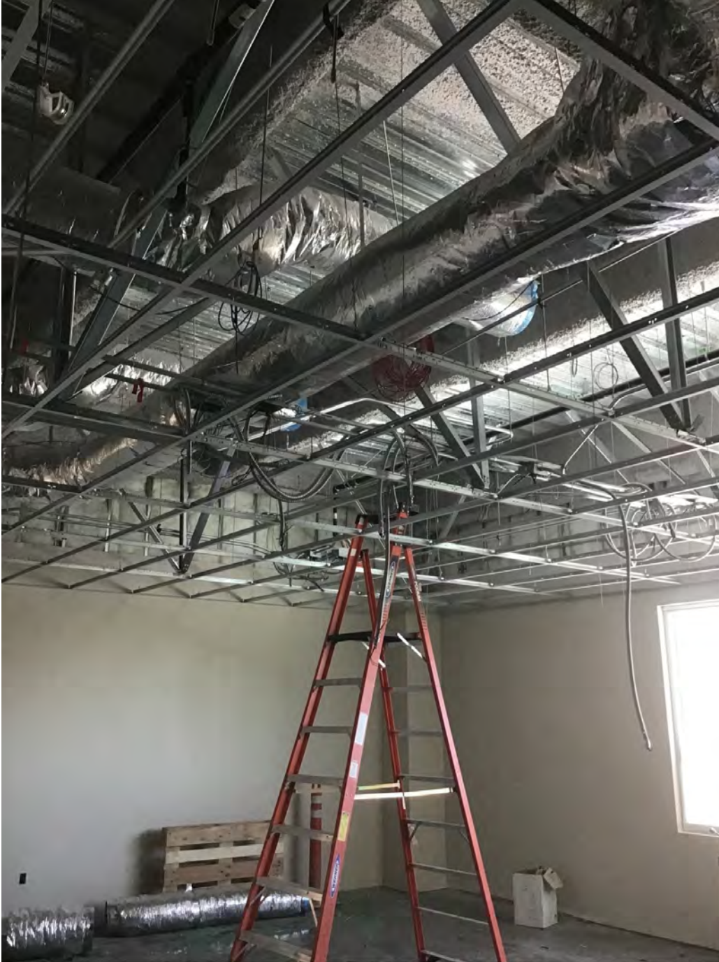
GRIDLOK® installed with conventional grid at Kindred/UC Davis using a post and two braces.
