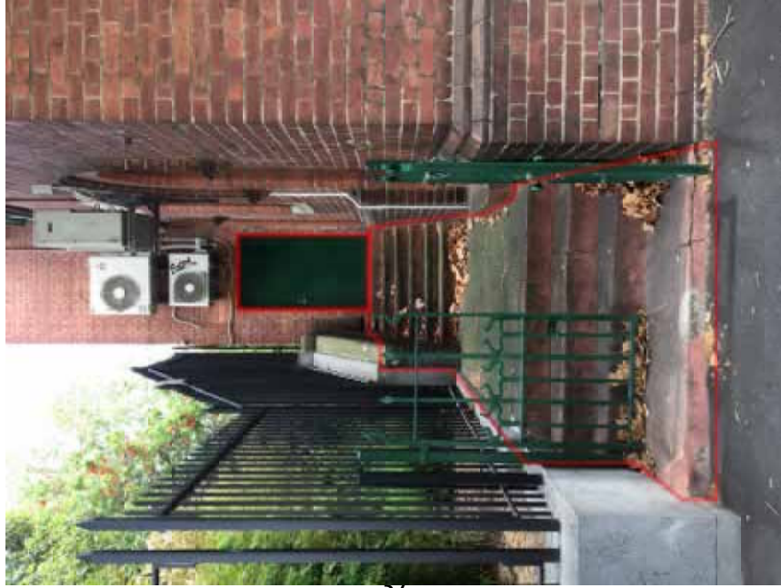
Figure 10: Proposed reconfiguration of existing stepped entrance from Gisborne street to provide a step free entrance.
