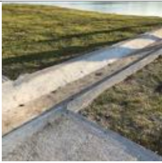
Photo 112. I-16 Drainage channels built at the viewing area on the north side of the Banje reservoir
