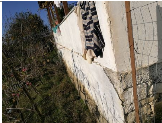
Photo 67. I-10 Water Stain on the Wall Showing the Flood Level
