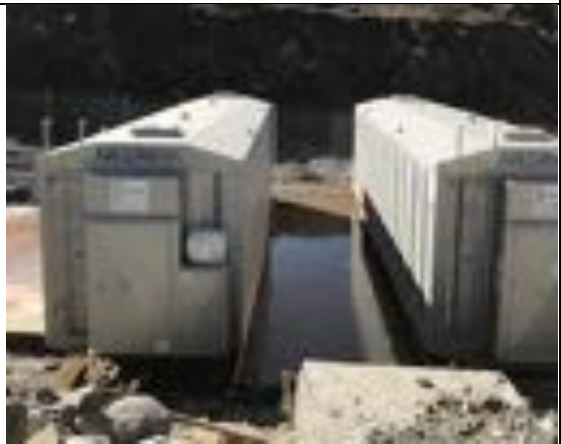
Photo 139. I-18 Arsimak wastewater treatment facilities at Moglice site camp
