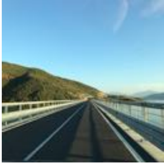
Photo 28. I-7 Close up of a bridge, part of the Banje-Gramsh replacement road
