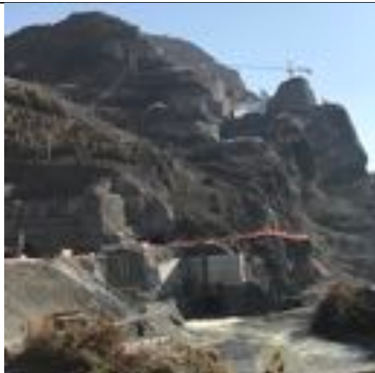
Photo 8. I-3 Right abutment of Moblice, with diversion tunnel at bottom centre of picture
