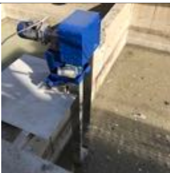
Photo 134. I-18 Oil skimmer at sediment pond
