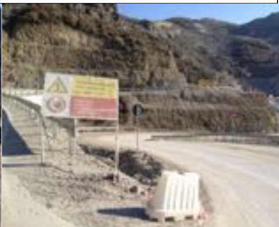
Photo 16. I-5 Entrance to Moglicë work site without access control
