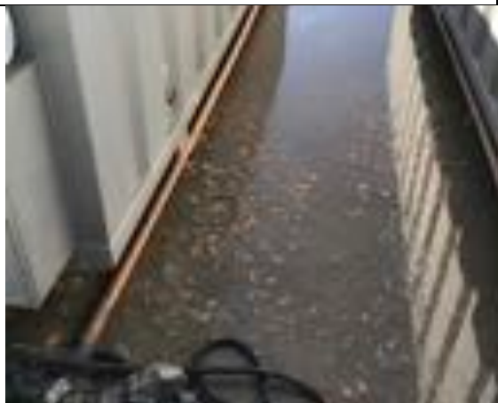
Photo 141. I-18 Sewage leaking or overflowing from Arsimak wastewater treatment plant
