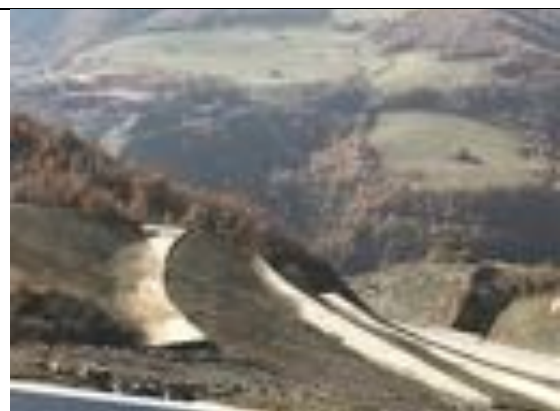
Photo 117. I-16 Concrete erosion-prevention terraces on the hillside above the Moglice construction site
