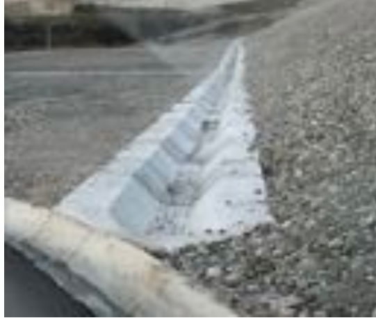
Photo 108. I-16 Example of a drainage channel, on the downstream face of Banje dam
