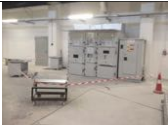
Photo 84. I-12 Restricted access to equipment
