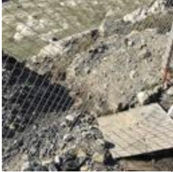
Photo 143. I-18 Overflowing sewage discharged to river
