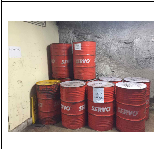
Photo 45: Temporary Storage of Turbine Oil in Powerhouse
