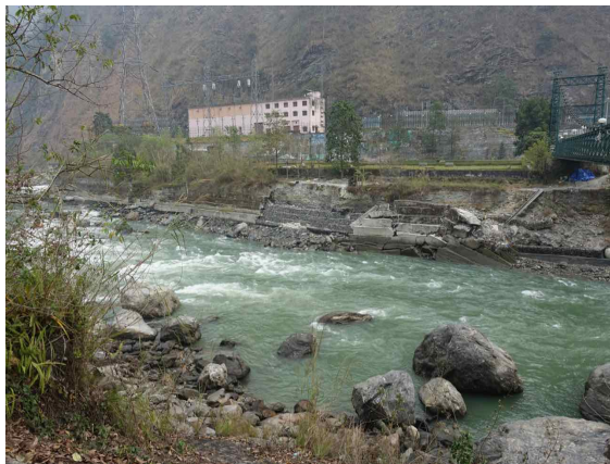
Photo 41: Teesta River at Powerhouse Showing Right Bank Protection Damaged by Boulders
