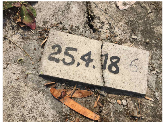
Photo 30: Monitoring of Cracks at Surge Shaft
