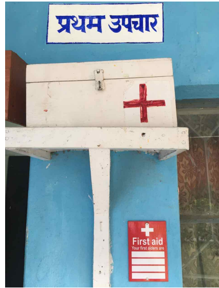
Photo 76: First Aid Equipment with Missing Information
