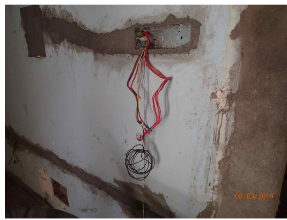
Photo 72: Electrical Safety Risk
