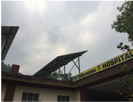
Photo 69: 800 kW Solar Project on Powerhouse Colony Hospital
