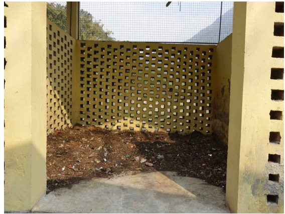
Photo 60: Solid Waste Stockpile Waiting Separation
