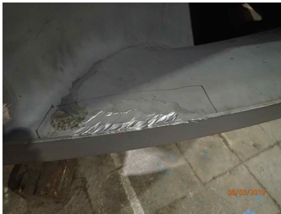
Photo 39: Erosion Damage to Runner
