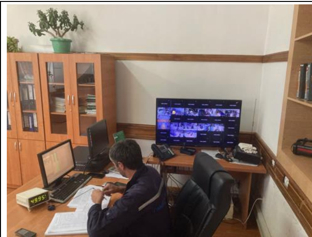
Photo 80: PEC control centre
