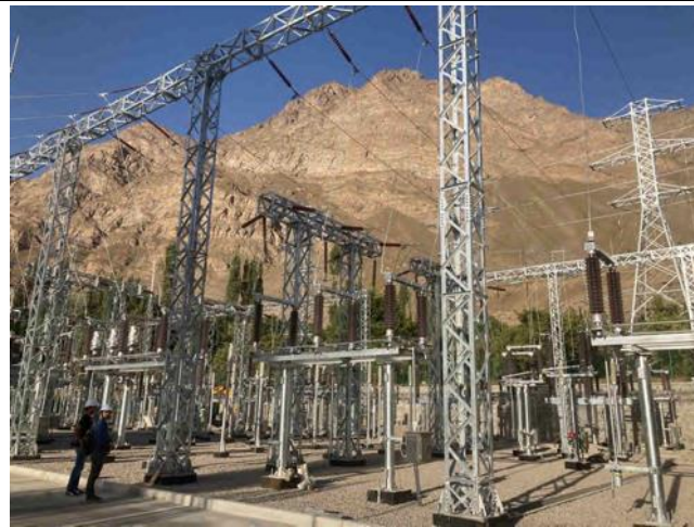
Photo 77: New 110kv substation at Khorog HPP
