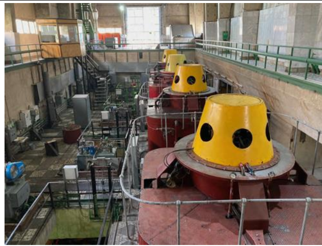
Photo 8: Pamir-1 HPP powerhouse
