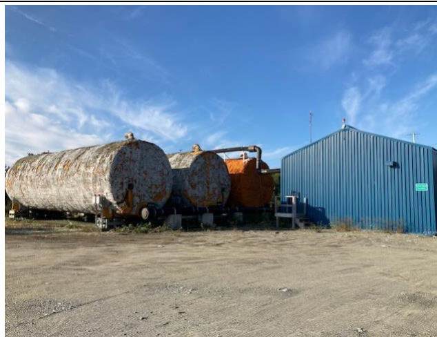
Photo 26: Insulated freshwater tanks
