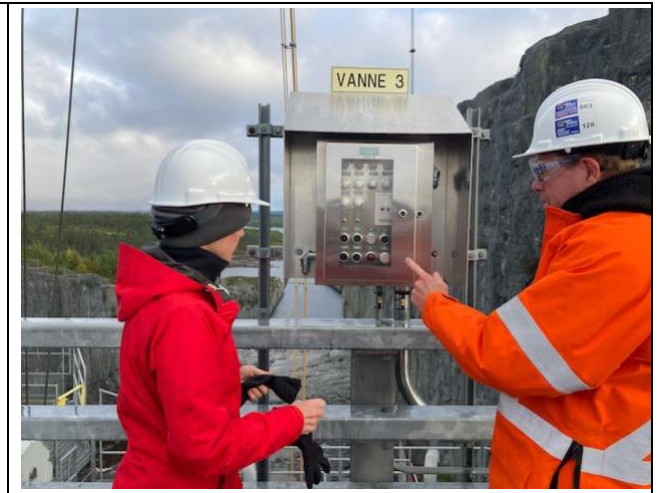
Photo 57: Spillway gate controls
