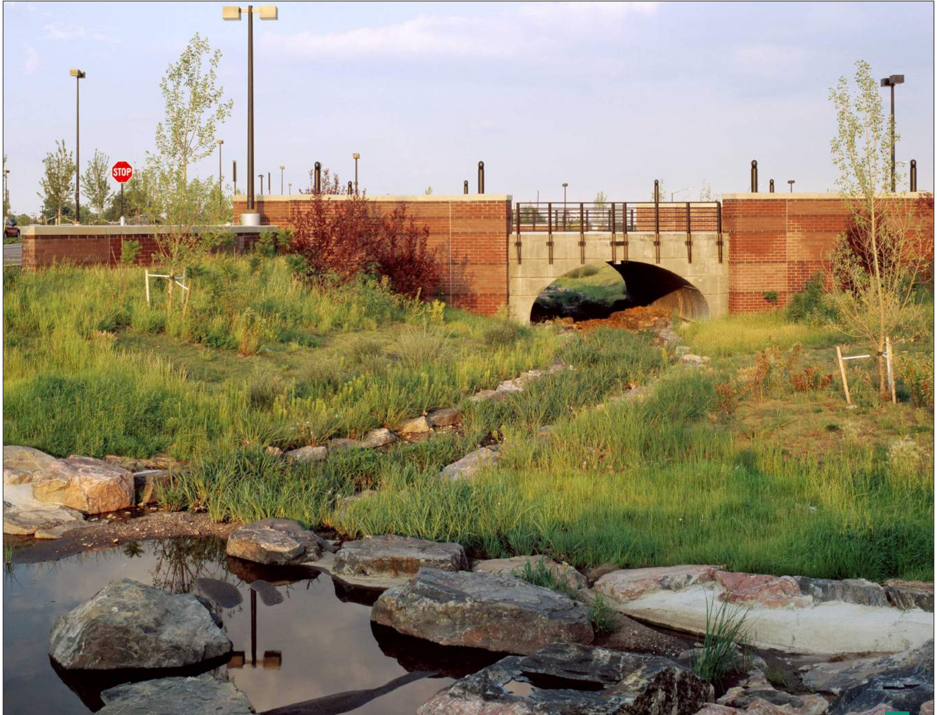
Dry Gulch Improvements at Colfax & Wadsworth / Photo Ken Papaleo, High Country Coloring
