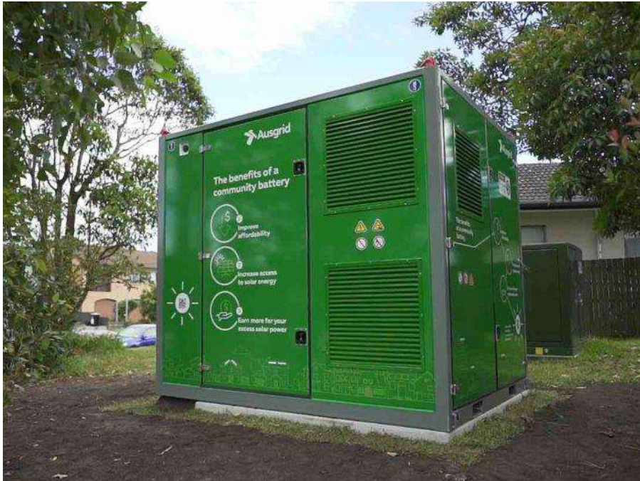
Figure 14 Ausgrid battery in New South Wales
