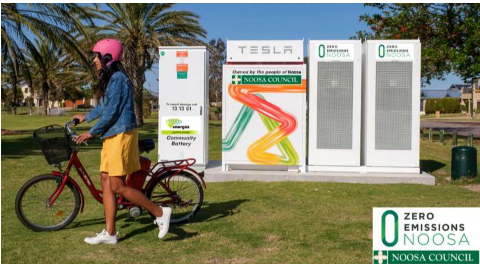
Image modified without permission from Western Power installation in WA.
