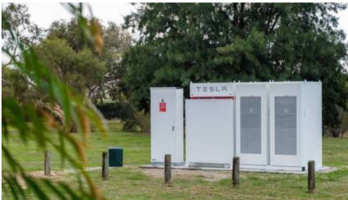
Figure 13 Powerbank installation in Western Australia
