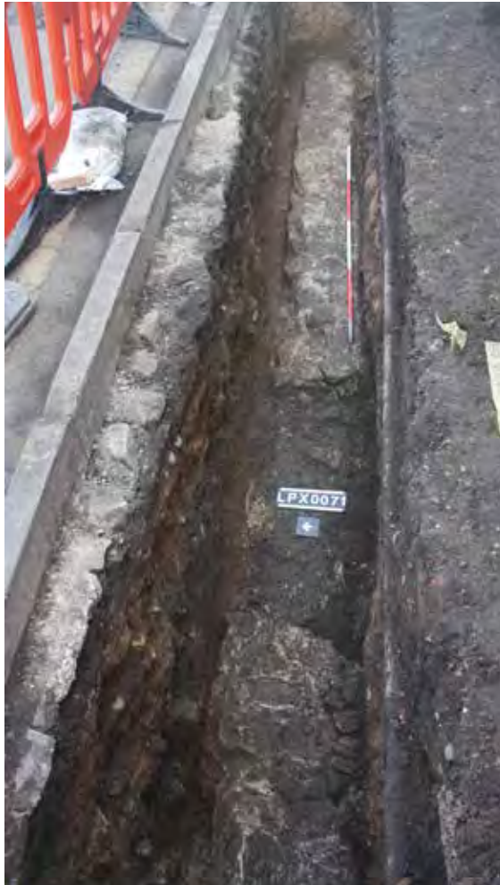
Cable Trench (1m wide) Looking west along the E-W aligned south wall of the northern cloister range, entrance way in mid ground.
