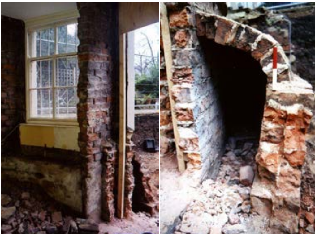
Left hand image - Interior view of wall 1218, window recess (left), brick vaulting 1081 (right)
