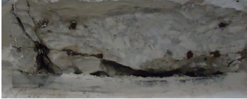
Figure 7: Cracking and spalling due to corrosion
