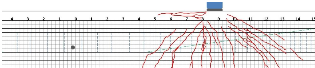
Figure 6: Shear test A2 cracking; strand rupture occurred at the 8-ft mark (3 in. grid shown)
