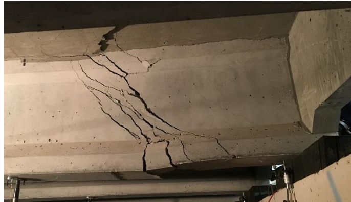
Figure 15: Final cracking in loaded bridge girder
