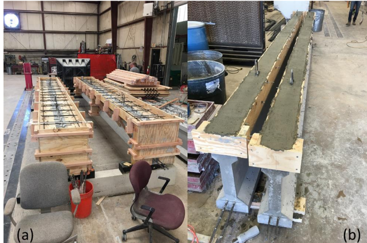
Figure 5: Completed scale girder specimens with sections of deck prior to and after casting
