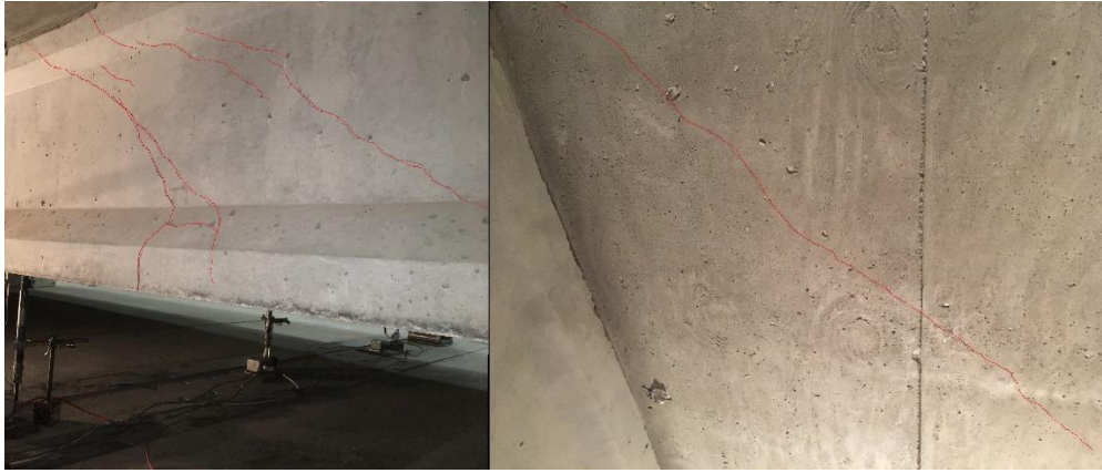
Figure 12: Bond shear cracking in loaded girder (left) and two way type cracking in deck slab (right)
