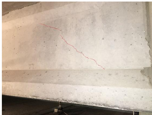
Figure 11: Initial crack during scale bridge test
