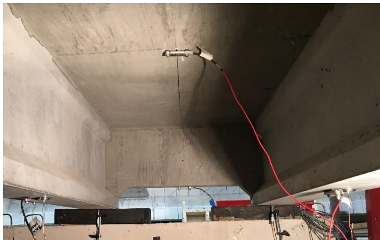
Figure 2: View from underneath scale bridge showing connection between girders and slab and the end diaphragm connection
