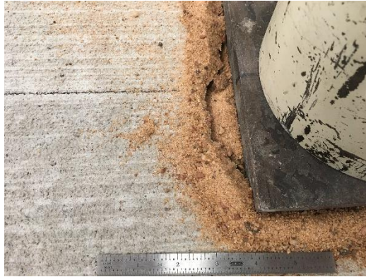
Figure 14: Punching shear failure in deck
