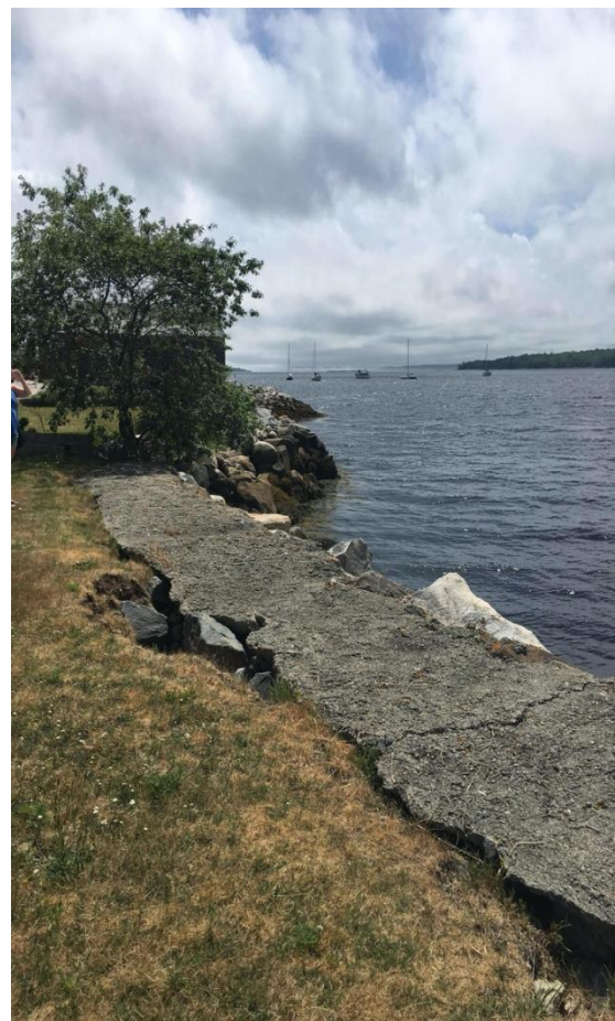
Figure 5. Scouring behind seawall. Note that the wall is lower in elevation than the land behind it (The Ecology Action Centre, n.d.)
