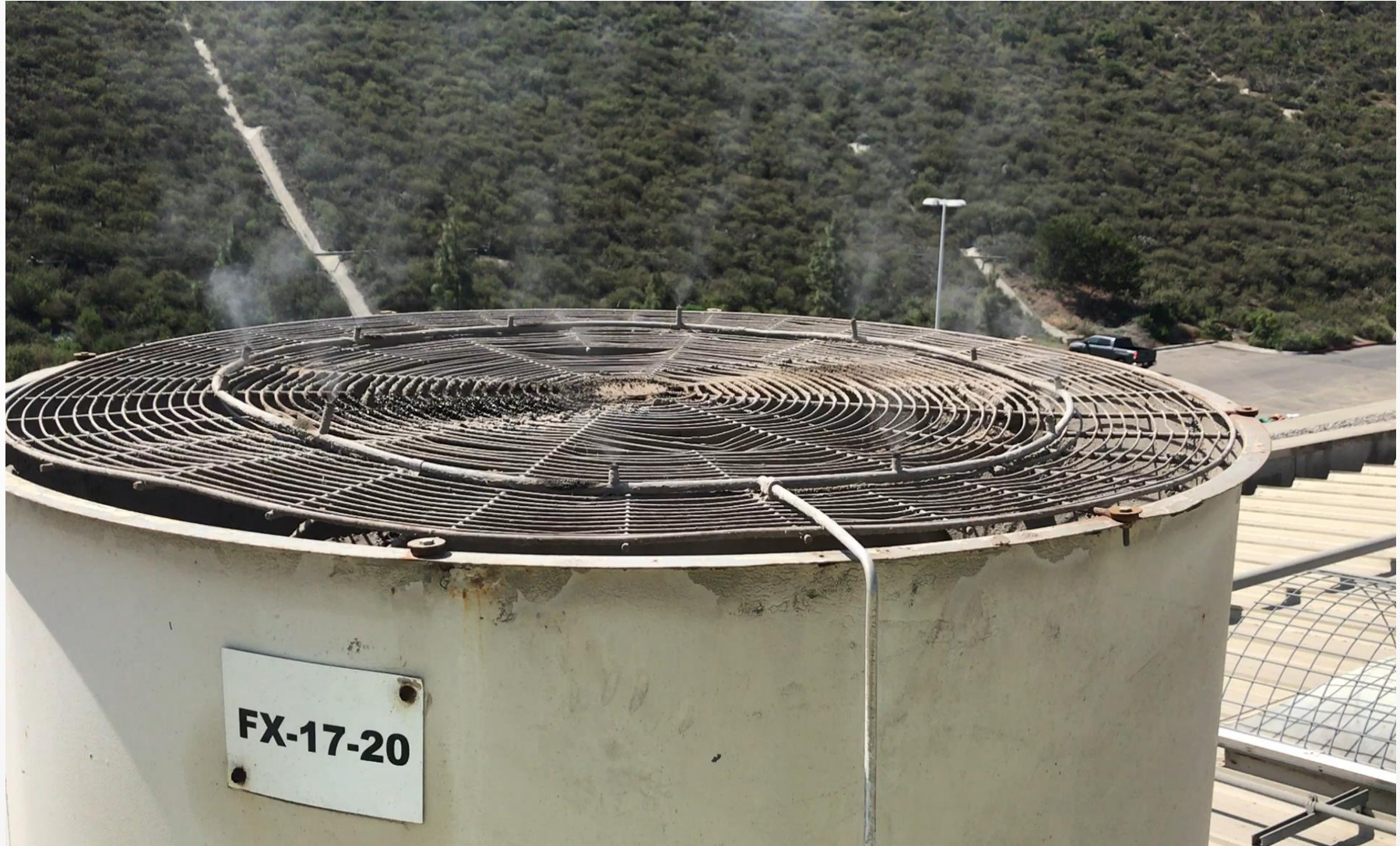
Chiquita Canyon WWT Plant aeration basin ( H_2S )
