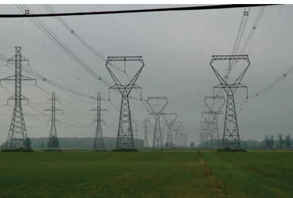
Figure 34: Transmission lines near Six Nations (photo credit: Power to the People, Real World Media)
