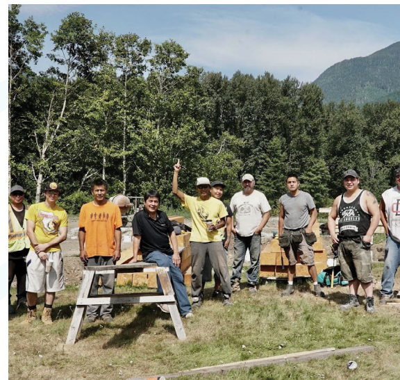
Figure 19: Community members in Bella Coola from the Nuxalk Nation working on energy efficient homes (photo credit: Power to the People, Real World Media)
