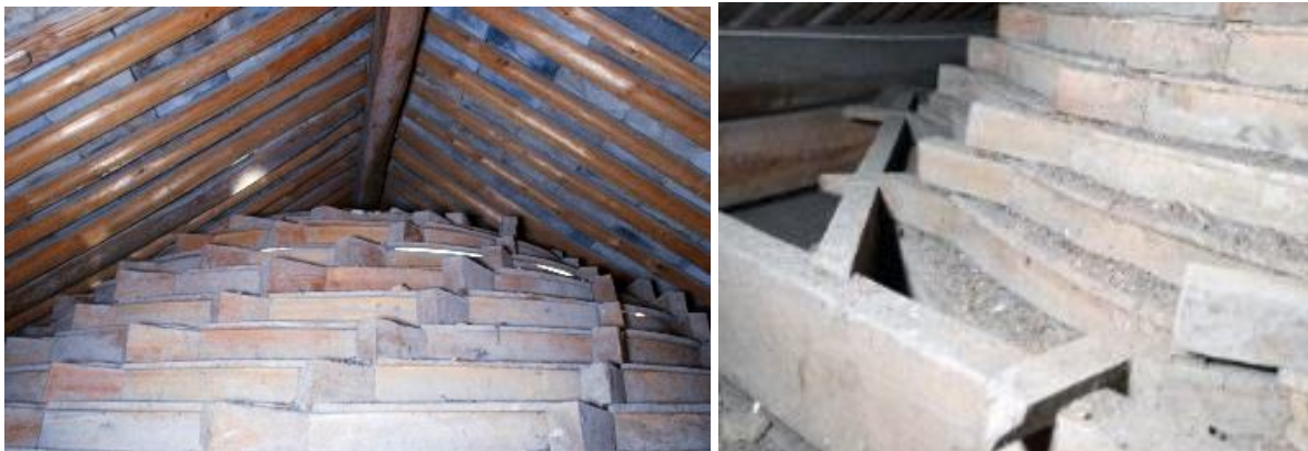
Fig. 11. The space between the roof and the spiral zaojing , built in the 1920s, in Ninghai. Ref. ZJ-01 © Jingxian Ye
