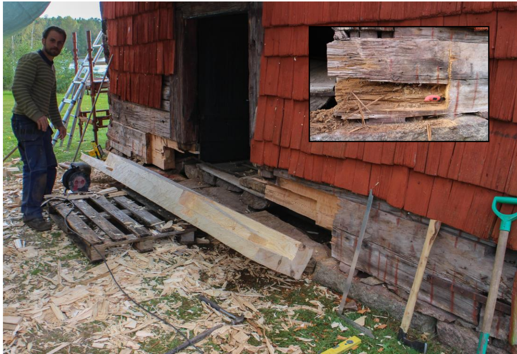
Fig. 4. Example of surgical repair of the front sill. The pasted photo shows the decay during cleansing. A pdf about the more complex conservation of the junction between tiebeam, rafter and wall plate can be found on the blog timmermanskonst.se . Photos Karl-Magnus Melin.
