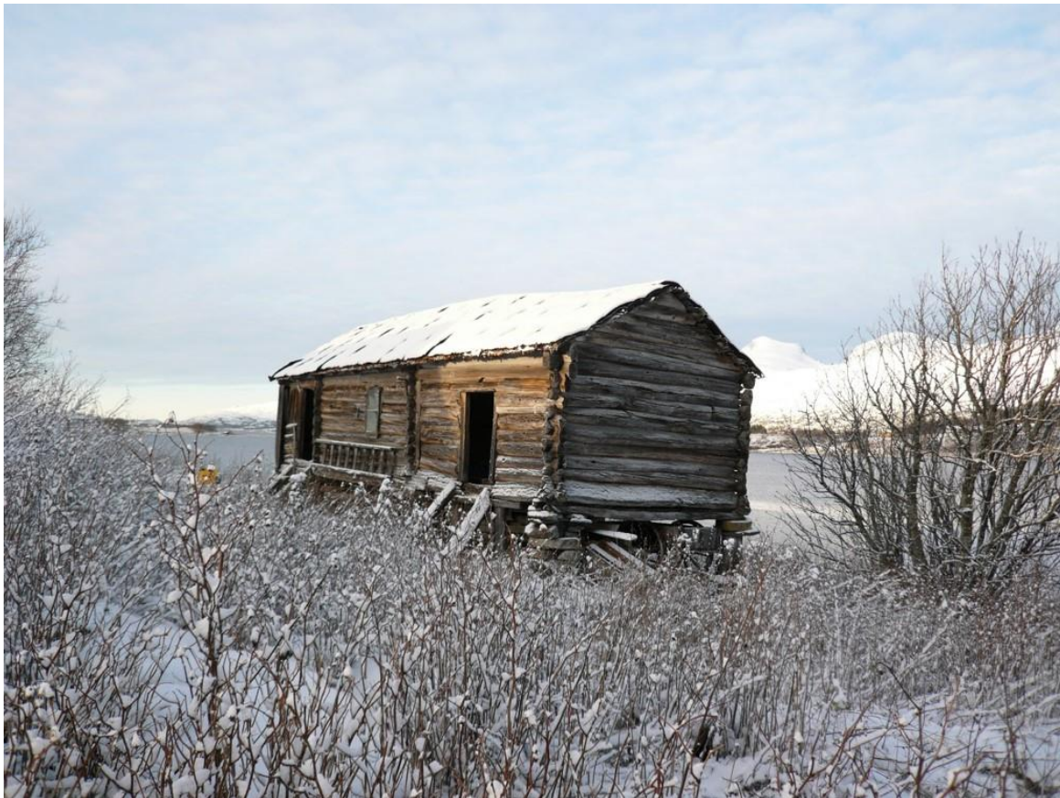
Fig. 8. Typical storhouse, dated 1637, with the short side orientated and twisted against the predominate wind. In the short wall against the southwest there is a timber frame «sval».
