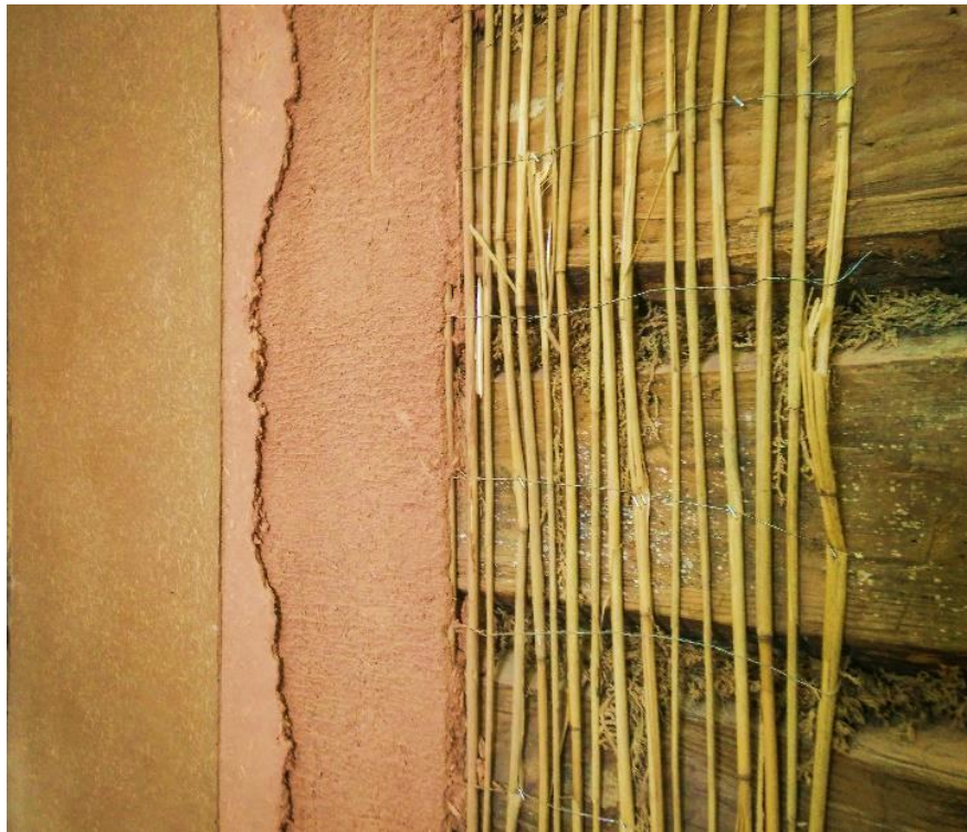
Fig. 4. Layers of clay plaster applied with a reed mat on a log wall. Photo: Indrek Kerbo
