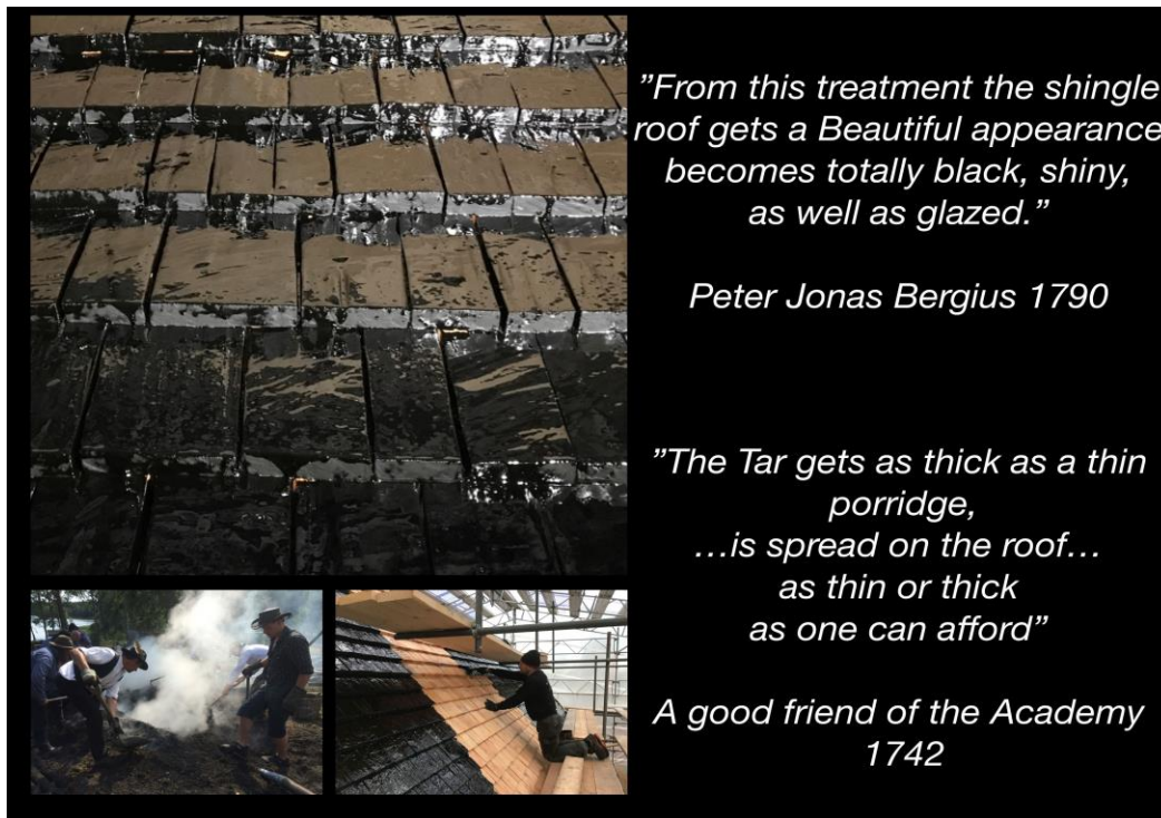
Fig. 7. Above, the shiny shingles after tarring. Below left the making of the tar. Below right, the tar is applied in "stripes" with minor changes of the recipes to be evaluated. Right citations from the used recipes.
