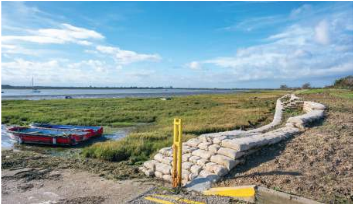
Two Tree Island. A green wall is being built to protect the island's coast from erosion.
