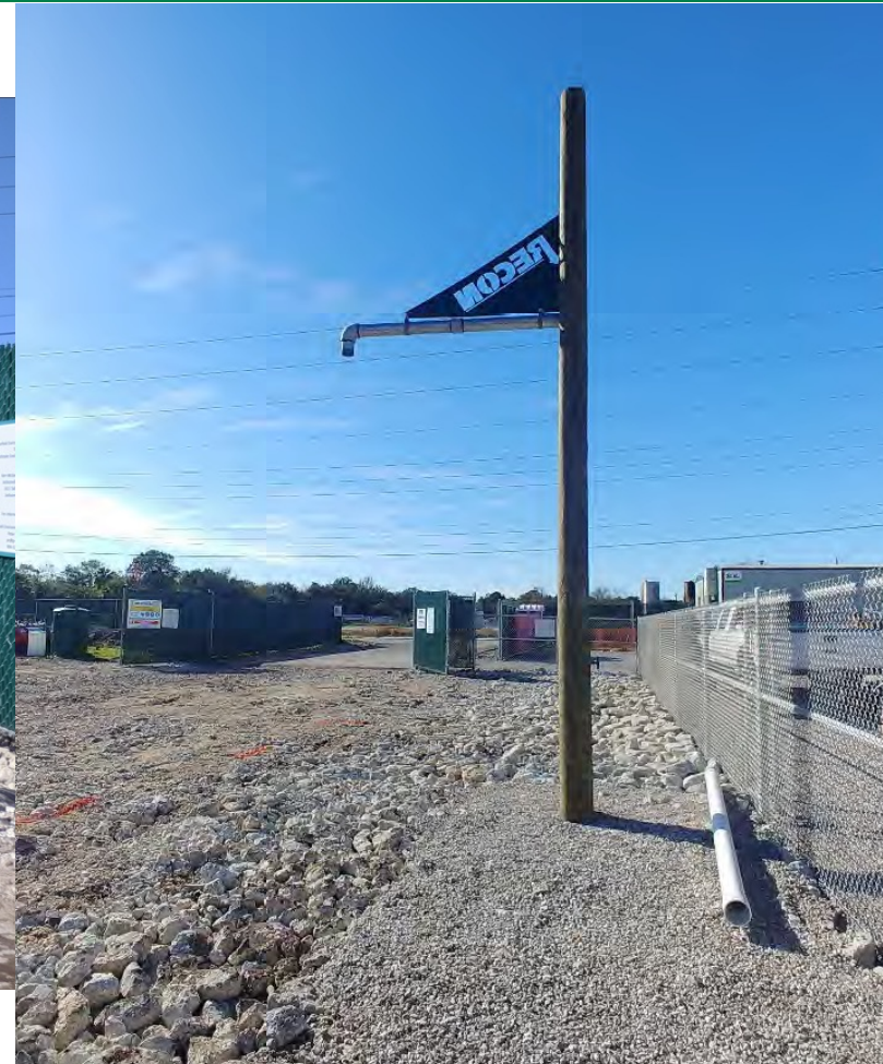
Water fill station and truck wash pad
