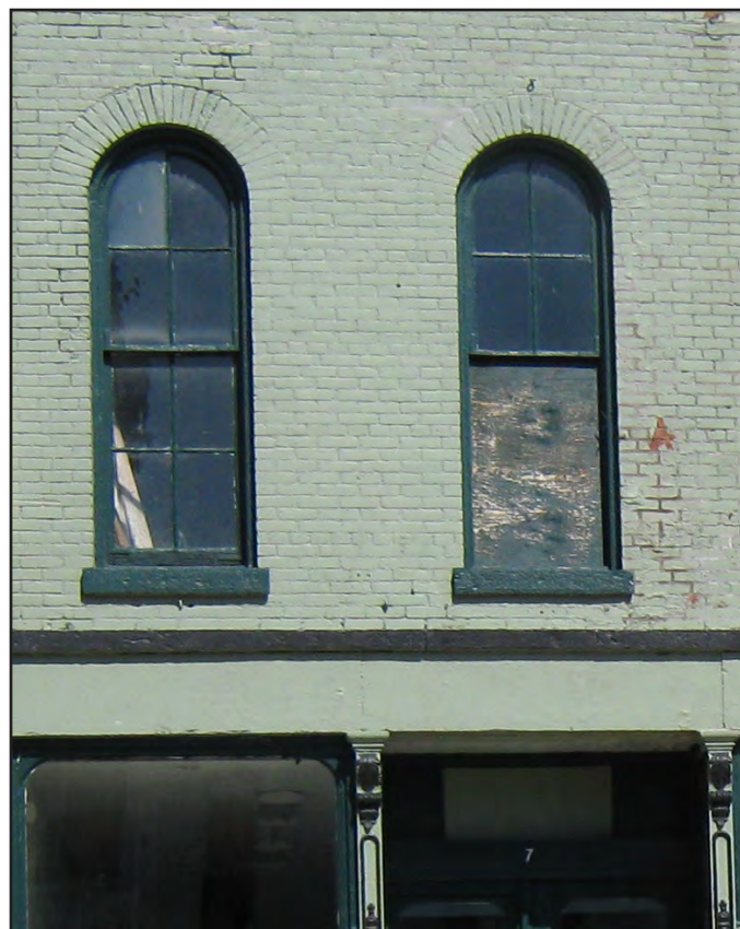
Vacant upper floor space in a village in the Genesee-Finger Lakes Region. (Photo - G/FLRPC)
