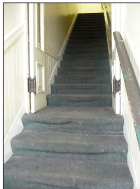
Frederick Douglass Apartments Stairways before repair. (Photo - Edgemere Development, Inc.)
