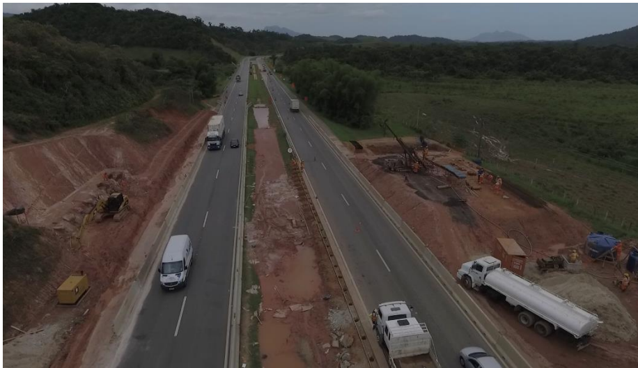
In November 2018, the corporation holding the toll-road concession began construction of Brazil's first forested wildlife overpass. The bridge will span BR101 highway.
