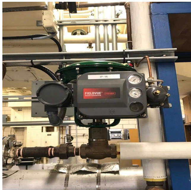
Figure 16. Valve FCV-39 used to activate steam flow
