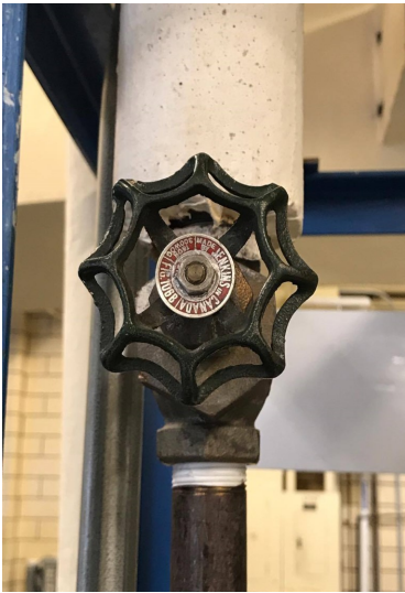
Figure 9. Steam Control Valve V-111
