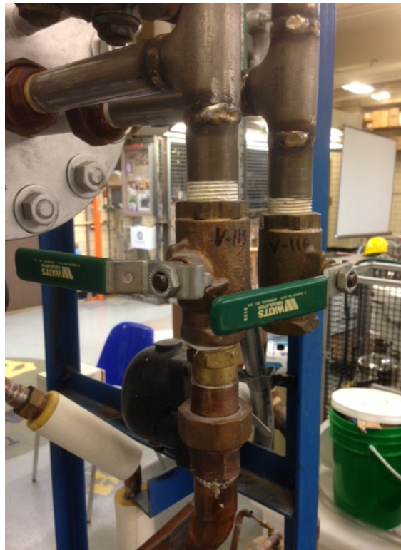
Figure 6. Cooling water drain valves V-115 and V-116
