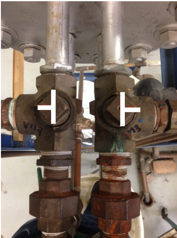
Figure 5. Cooling water control valves V-112 and V-113
