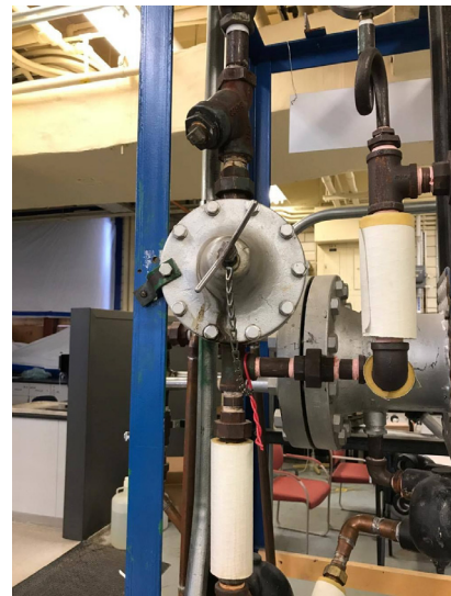
Figure 10. Pressure Reducing Steam Valve PRV-10
