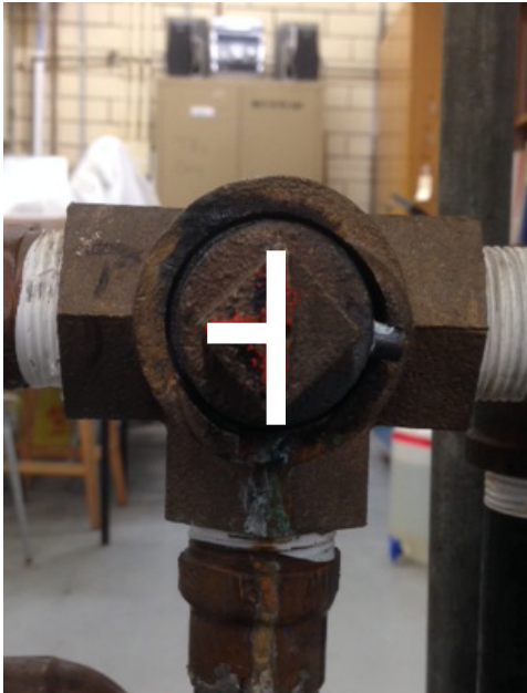
Figure 22. Three-way valve V-122 for cooling water flow
