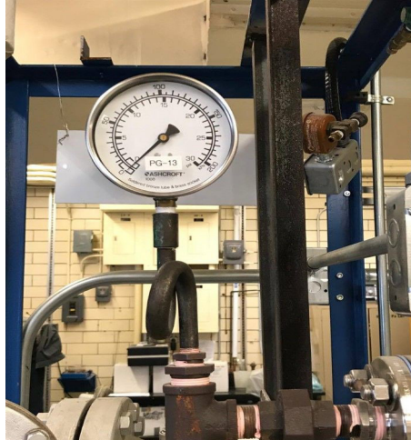
Figure 17. Steam Pressure gauge PG-13
