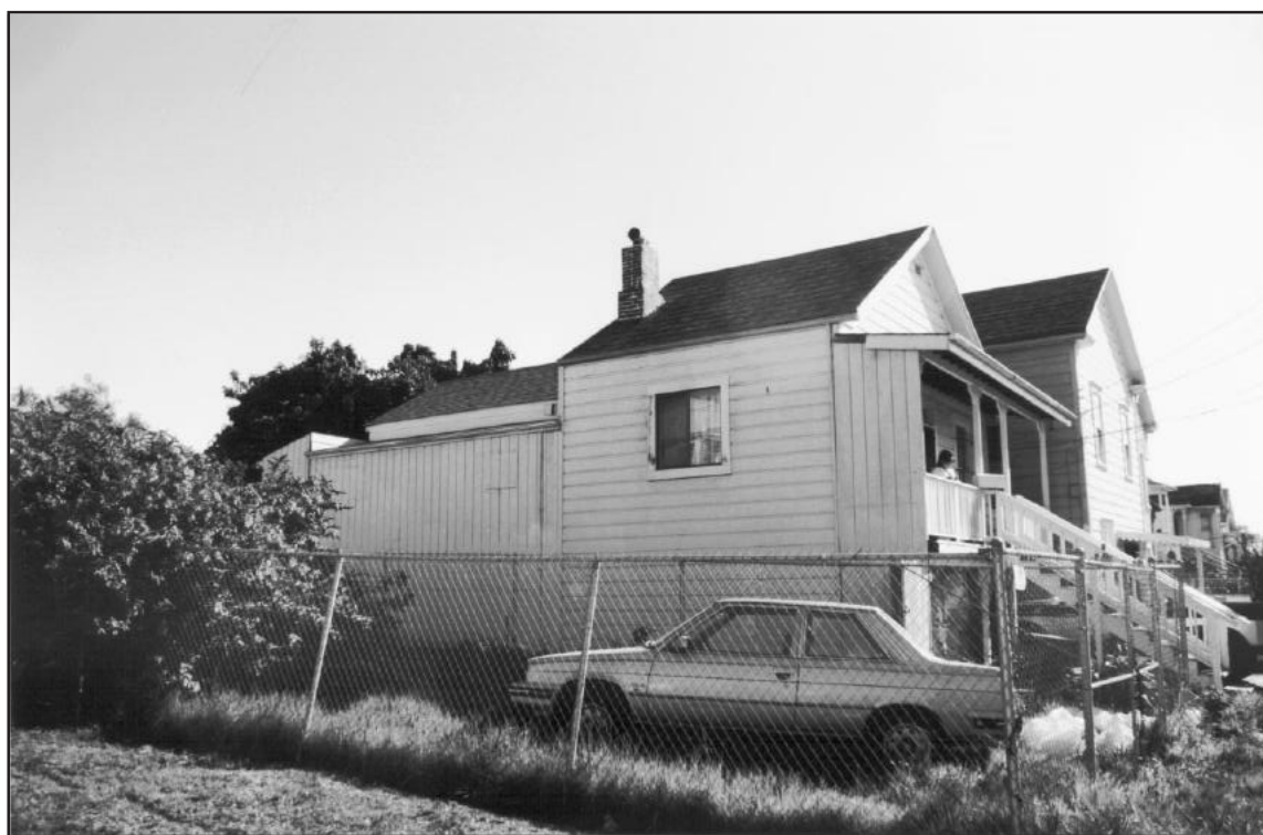
PLATE 30. SIDE ELEVATION OF SUGRUE/CROSSMAN COTTAGE, 360 CHESTER STREET. The three phases of addition to the back of the building clearly show. The chimney and the higher roof indicate the end of the original two-room house. The lower gable roof (towards the back of the picture) shows a later addition. The parts of the building clad in vertical siding indicate the newest additions. (Credit: Paul Groth)
