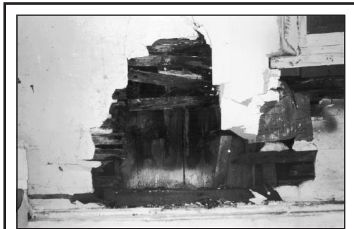
PLATE 11. DETAIL OF SINGLE-WALL CONSTRUCTION IN THE KITCHEN OF 714 PINE STREET. The wide vertical boards are the exterior structural wall; the horizontal lath and its covering of plaster help to seal the wall. Note the corner of a window sill at the upper right. (Credit: Marta Gutman)
