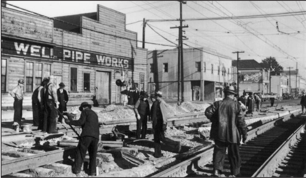
PLATE 81. LAYING TRACK ALONG SEVENTH STREET FOR THE NEW RED TRAIN SERVICE IN 1938. There appear to be plenty of workers and onlookers as the new tracks were laid for the passenger service over the Bay Bridge. While this was a one-time event, maintenance and repair of streets and railroad tracks kept some individuals employed year-round. The Well Pipe Works occupies a building that advertised metal works in the 1880s; both would have kept a small contingent of workers employed. Across the street on the corner was the former Centennial Hotel (the Astoria Hotel at the time of this photo), whose corner bar provided solace and entertainment for off-duty workers in the neighborhood. (From the collection of Vernon J. Sappers)
