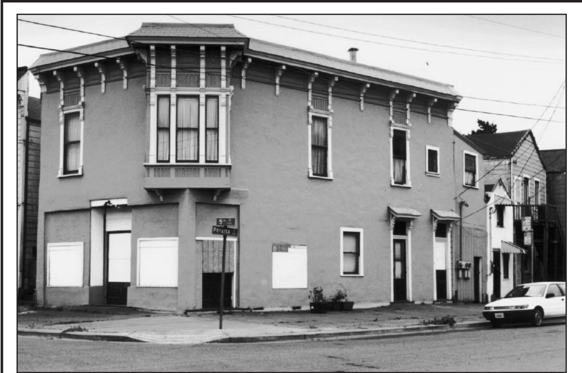
PLATE 40. CORNER VIEW OF THE DAVIDSON/PATTERSON STORE AND ROOMING HOUSE AT FIFTH AND PERALTA STREETS. The front door, at 1619 Fifth, leads into the former saloon and store. The two side doors with small hood roofs, at 370-372 Peralta, are the entry to the back of the store and to the upstairs rooming house. Davidson's shed and flats are visible on Peralta Street, behind the main building. (Credit: Paul Groth)
