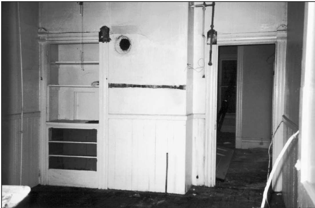
PLATE 22. NORTH WALL OF KITCHEN AT 1817 SHOREY STREET. Left, the butler's pantry reduced to storage shelves and drawers with a pass-through. Right, the door to the dining room, with pipes indicating former location of the hot-water heater. The range would have stood at the center. (Credit: Marta Gutman)
