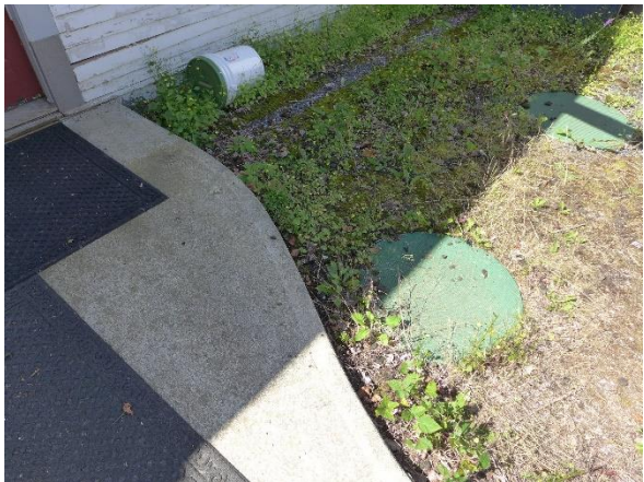
Fig. 5: Pump vault lids adjacent to N. patio slab & side double door, store entrance.
