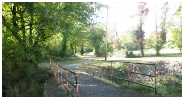
Greenway Bikeway: Existing bridge railings do not meet current standards and should be upgraded.
