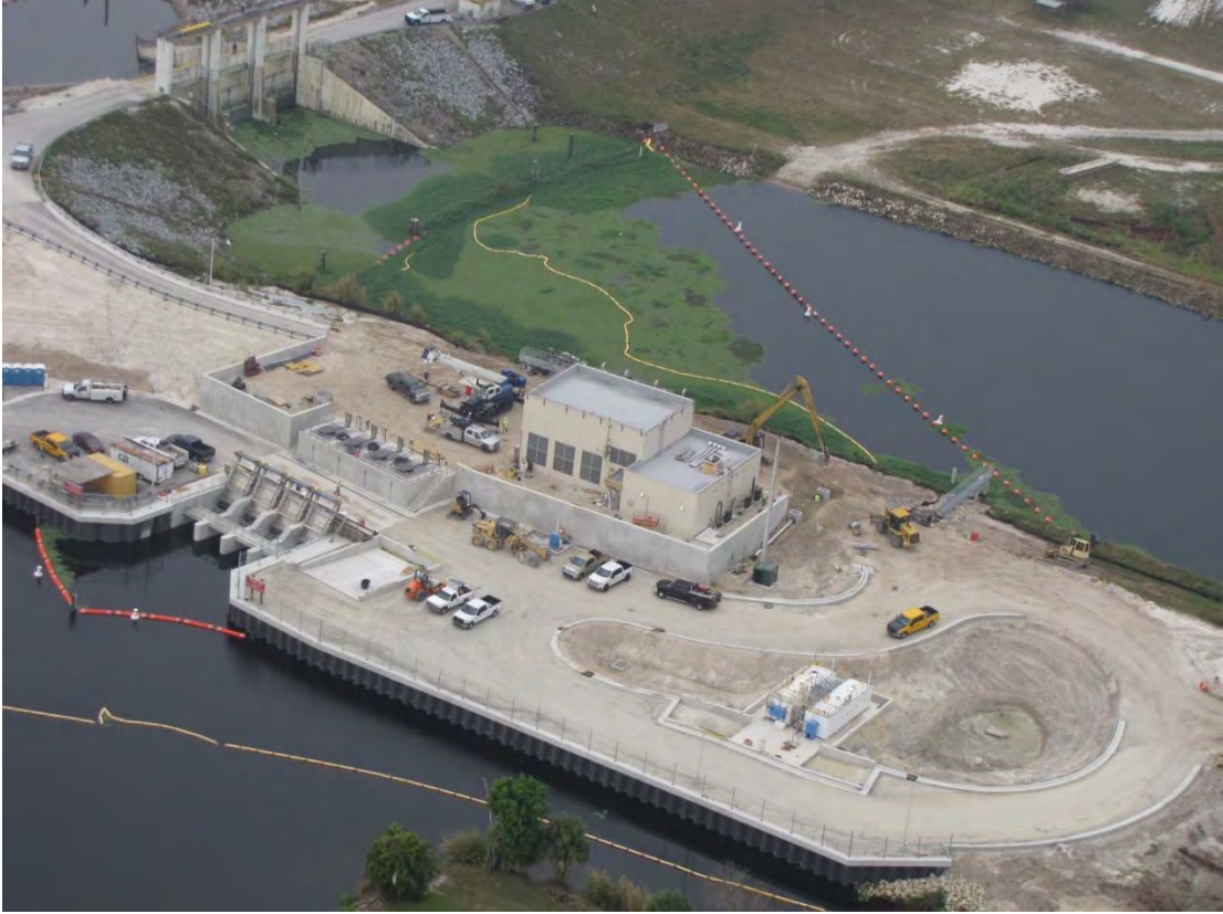
Lakeside Ranch Phase III – S-191A Pump Station
