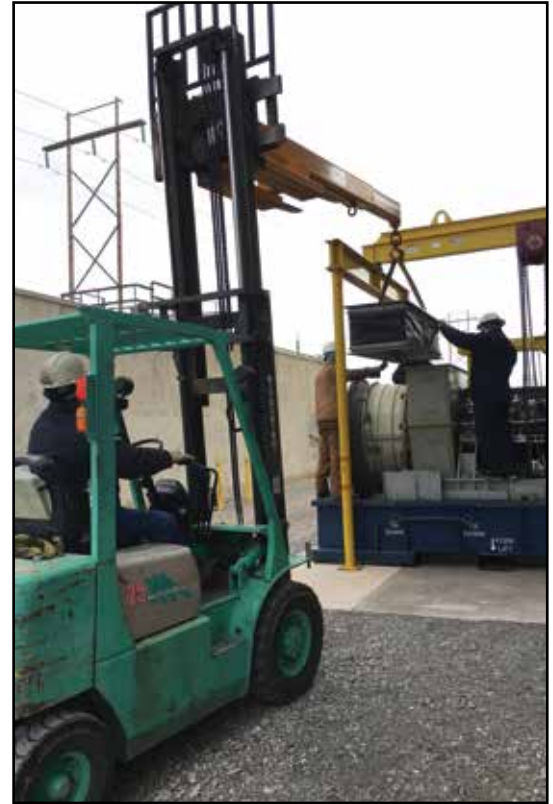
Randy Ryans, a mechanic at WFEC's Anadarko Plant, assists a contractor with unloading engine parts during recent outage.
