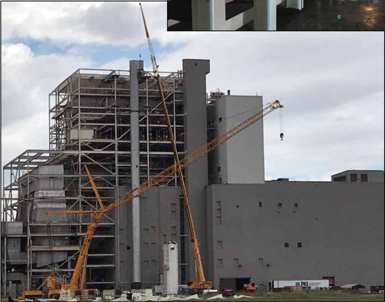
In order to make room for the new system, it was necessary to demolish the existing bottom ash system and existing auxiliary boiler. Removal required the use of large cranes to reach the affected areas.
