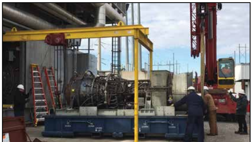
On-site contract crews, assisted by plant personnel, position Unit 8's engine, in preparation of installation at the Anadarko Plant.
