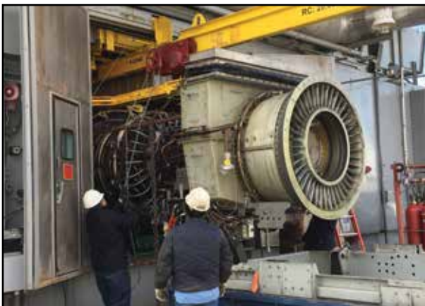
Installing Unit 8's engine after being returned to the Anadarko Plant following repair work in Dallas.
