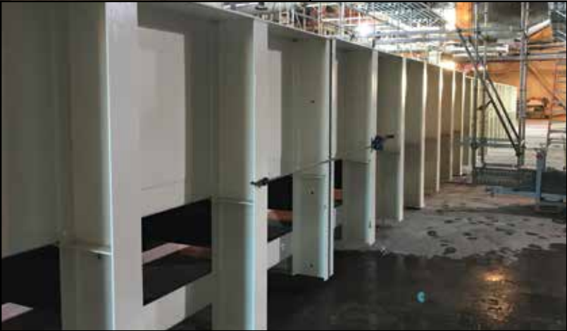
A conveyor belt trough was installed during the outage, as a part of the overall new conveyor system.
