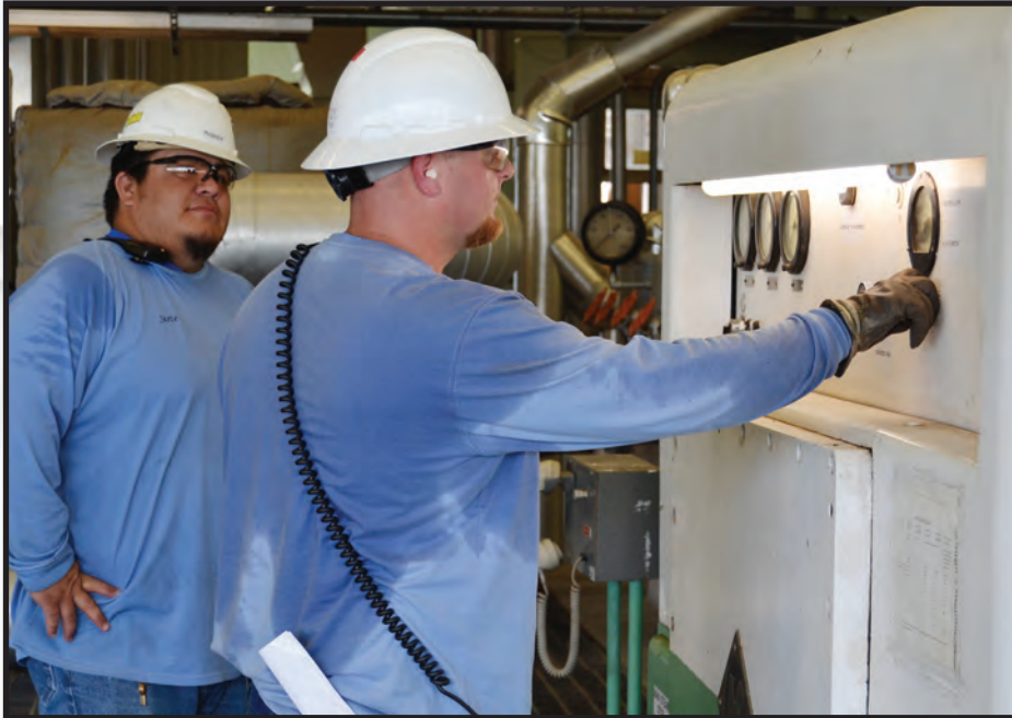
Relief Shift Supervisor Eric Ladyman (front) adjusts the steam admission valves to “stretch” the turbine prior to rolling up to synchronous speed. Relief Auxiliary Operator Steve Mopope observes this phase during the annual operational testing on Anadarko Unit 3.
