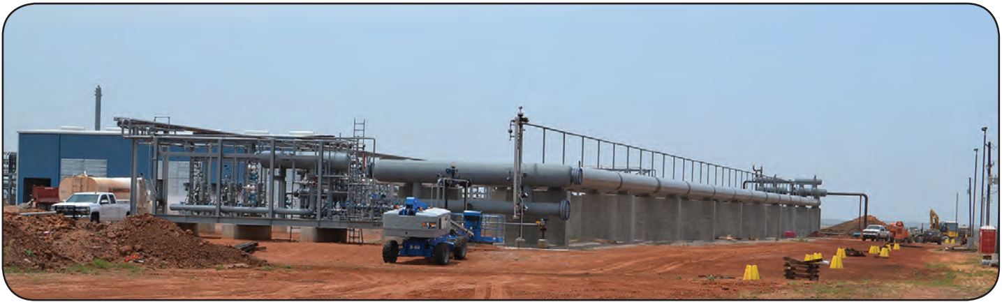
The MarkWest Omega Plant (shown above), has been constructed to accommodate the oil and gas growth in Cimarron Electric's service territory. MarkWest has plans to expand this current plant in the future. There are also other loads coming online in the future in other areas of Cimarron Electric's system. The MarkWest Plant is processing product from the area.
