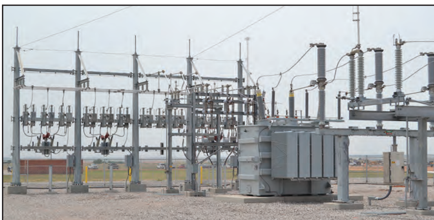
WFEC has constructed three new substations to accommodate load demands in this area. Pictured above is the newly constructed Park Community Substation, located in Kingfisher County, west of Okarche. This 138/26.4 kilovolt substation has three equipped circuits and one spare to serve the MarkWest Omega Plant, plus the growing oil load in the area.
