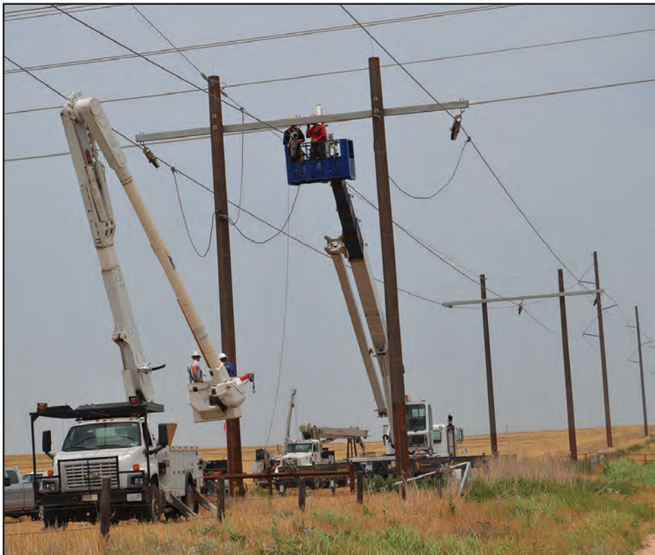
Crews from Maslonka Powerline Services, from Spokane, Wash., are shown constructing transmission lines in Cimarron Electric's service territory. This project consists of approximately 11 miles of new 138 kilovolt transmission line from the new Park Community Substation to the Kingfisher Switch Station.
