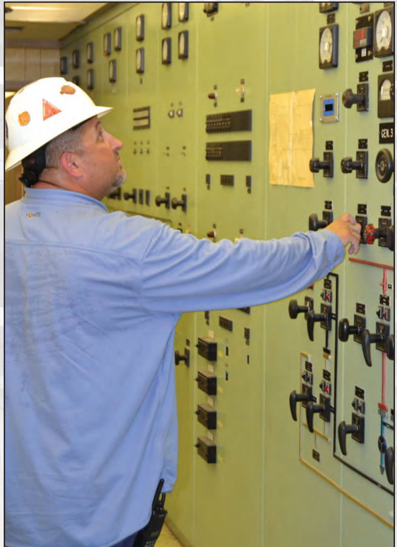
Relief Control Room operator Mike Anderson (right) adjusts voltage to match system conditions prior to closing the main generator breaker. This work was performed during a recent test of Anadarko Unit 3.
