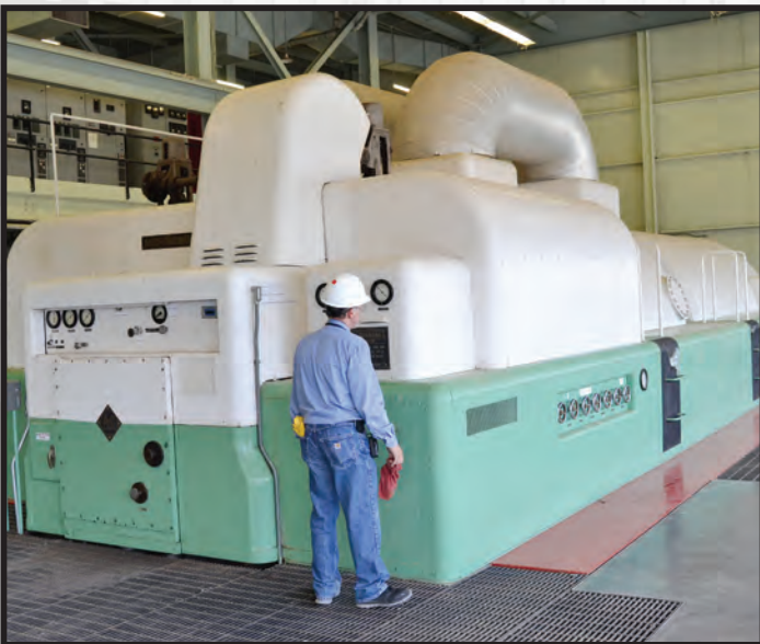
Anadarko Plant Maintenance Superintendent Clem Cassmeyer monitors sealing pressure steam at Unit 3 front standard. Sealing steam prevents air leakage and vacuum loss around the turbine shaft.
