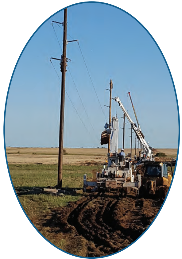
WFEC crews repair damage from widespread storms that occurred in mid-May. The top photo was taken on the Hulen Tap Line, while the bottom photo shows crews removing debris on the Morewood SW to Elk City PSO line. Three storms caused significant damage in a combination of 13 counties within WFEC's service area with a total of 206 structures requiring replacement or repair.
