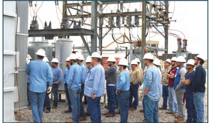
Switch training with new WFEC and member distribution cooperative power line employees is hosted annually.
