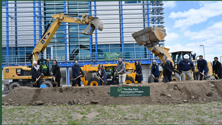
On Earth Day 2021, Governor Andrew M. Cuomo announced the start of construction for the Bay Park Conveyance Project Source: Kevin P. Coughlin / Office of Governor Andrew M. Cuomo
