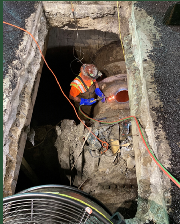
Crews work to open the aqueduct at Pit Q to inspect and survey the condition of the pipe
