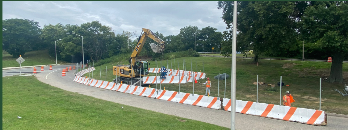
MPT is set at Pit A/Bay Park Shaft 9 located at the Sunrise Highway/Merrick Road (Photo: August 2021)
