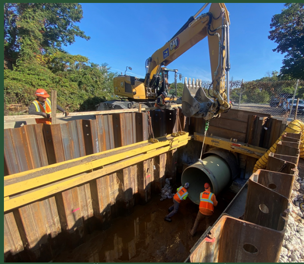
Crews installing a test pipe within the existing aqueduct at Pit P (October 2021)
