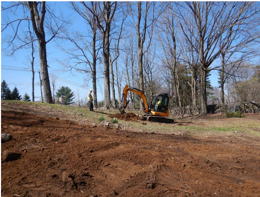
Photo 12. Backhoe mechanically excavating Trench 2 along the rise to determine how the landscape has been altered through time.
