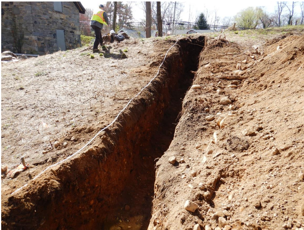
Photo 2. 10-meter mechanical trench excavated into the side of the raised hill in the western portion of the study area to examine the stratigraphy.
