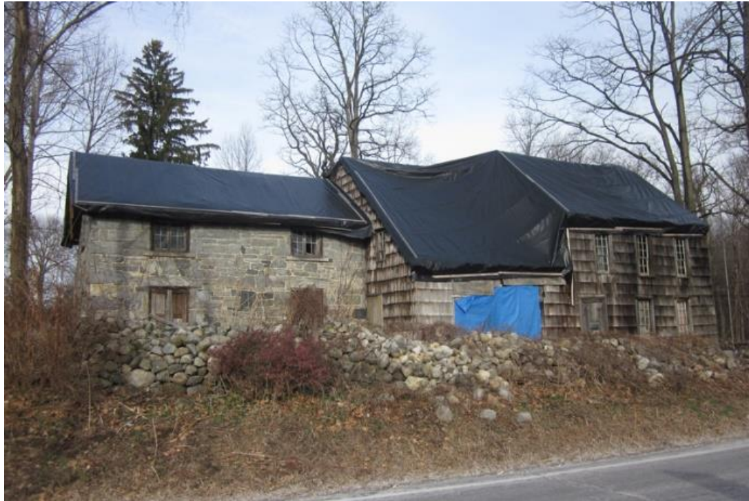
Figure 22. North facing view of the Odell House from Ridge Road. Tarps cover the roof to protect the structure from further damage. Original construction is centrally located with the steeper sloping roof.
