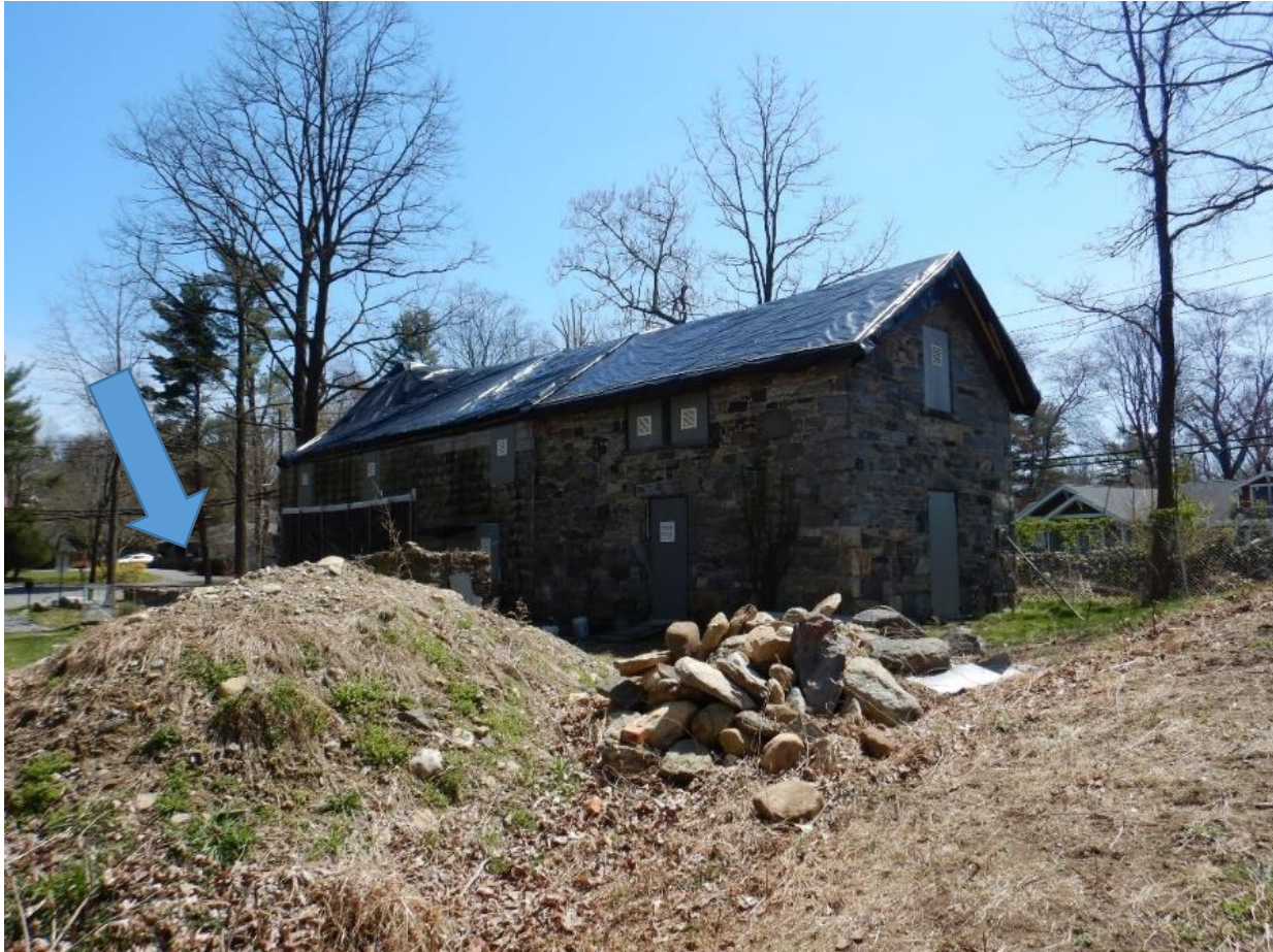
Figure 28. A view to the southeast of the rear of the house with a spoil pile from the interior on the left, and larger stone and concrete pile to the right.
