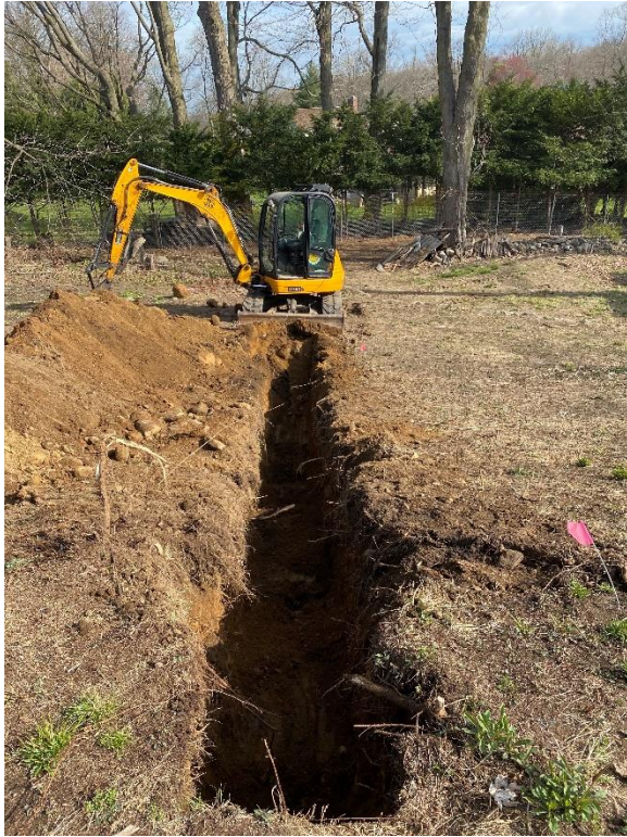
Photo 15. Completed excavation of Trench 1 with a backhoe provided by the Town of Greenburgh, 10x1 meters.
