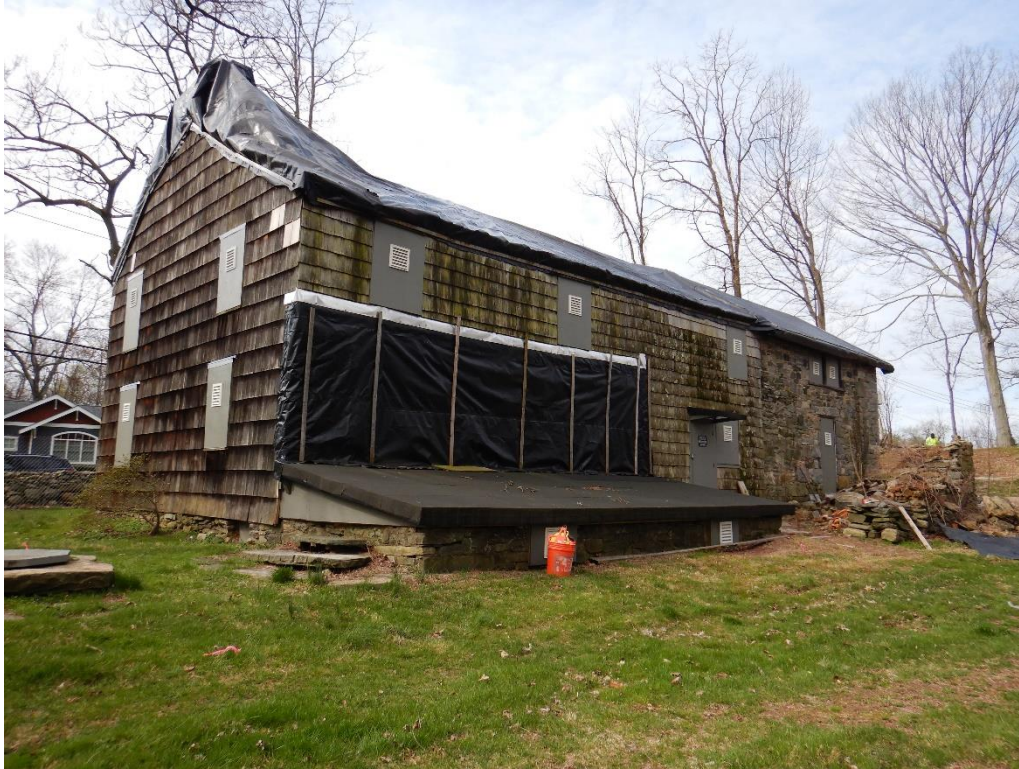
Photo 1. Rearview of the Odell House Rochambeau Headquarters with the original structure (1732) centrally located, the second wooden addition (1765) located in the left side of the photo, and the later stone addition (1855) on the right portion of the photograph.
