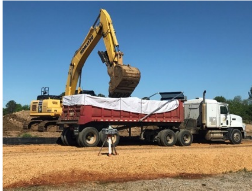
Photograph of Excavation Remedial Action at Kerr-McGee Superfund Site in Columbus, MS
