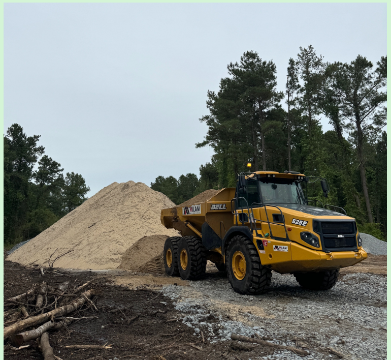
Loading clean fill from a staging area on Site in May 2024, as part of the Operable Unit 2 cleanup work
