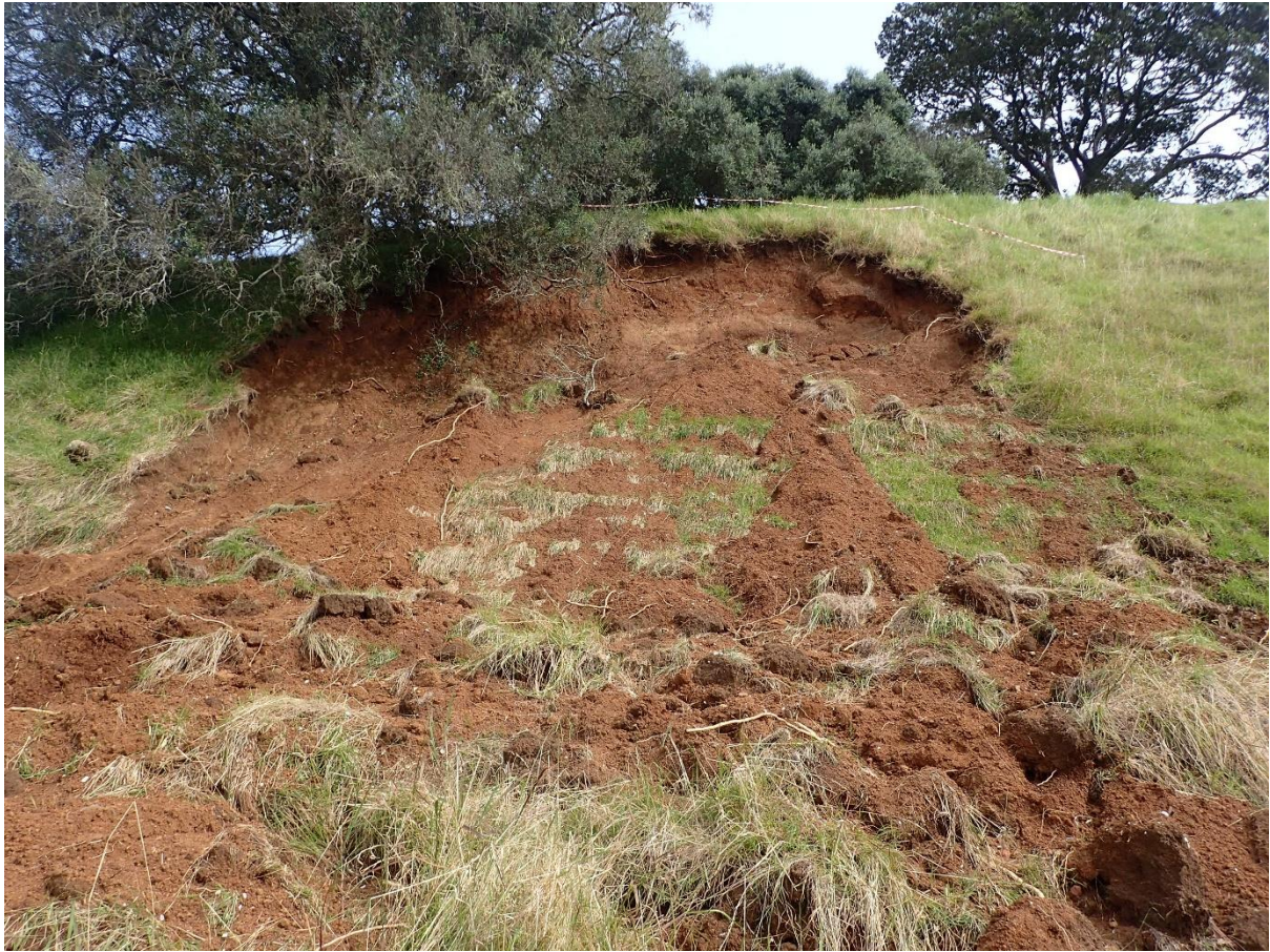
Fig. 12. Looking up slip 12 which is a slope failure on the riser between two terraces.
