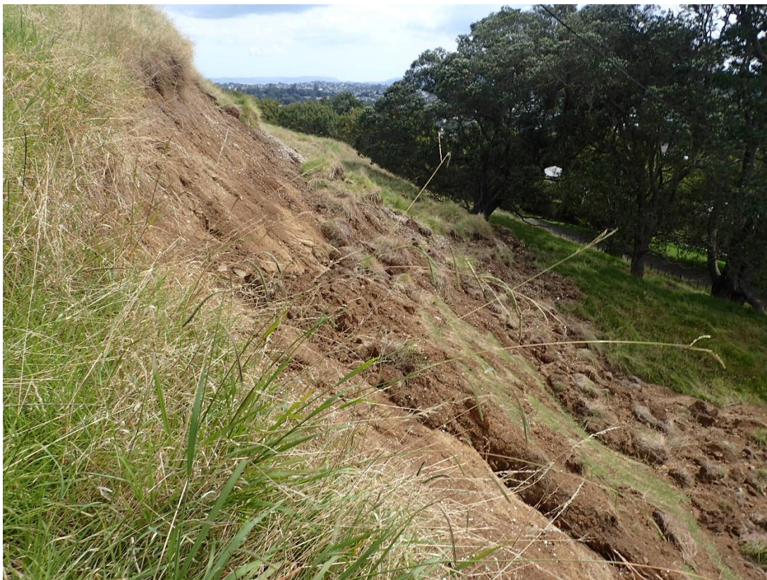
Fig. 7. Slip 6 shows the over steepened nature of the slope that failed and the shallow depth of regolith that has flowed down slope like a carpet of grass and topsoil developed in the terrace fill.
