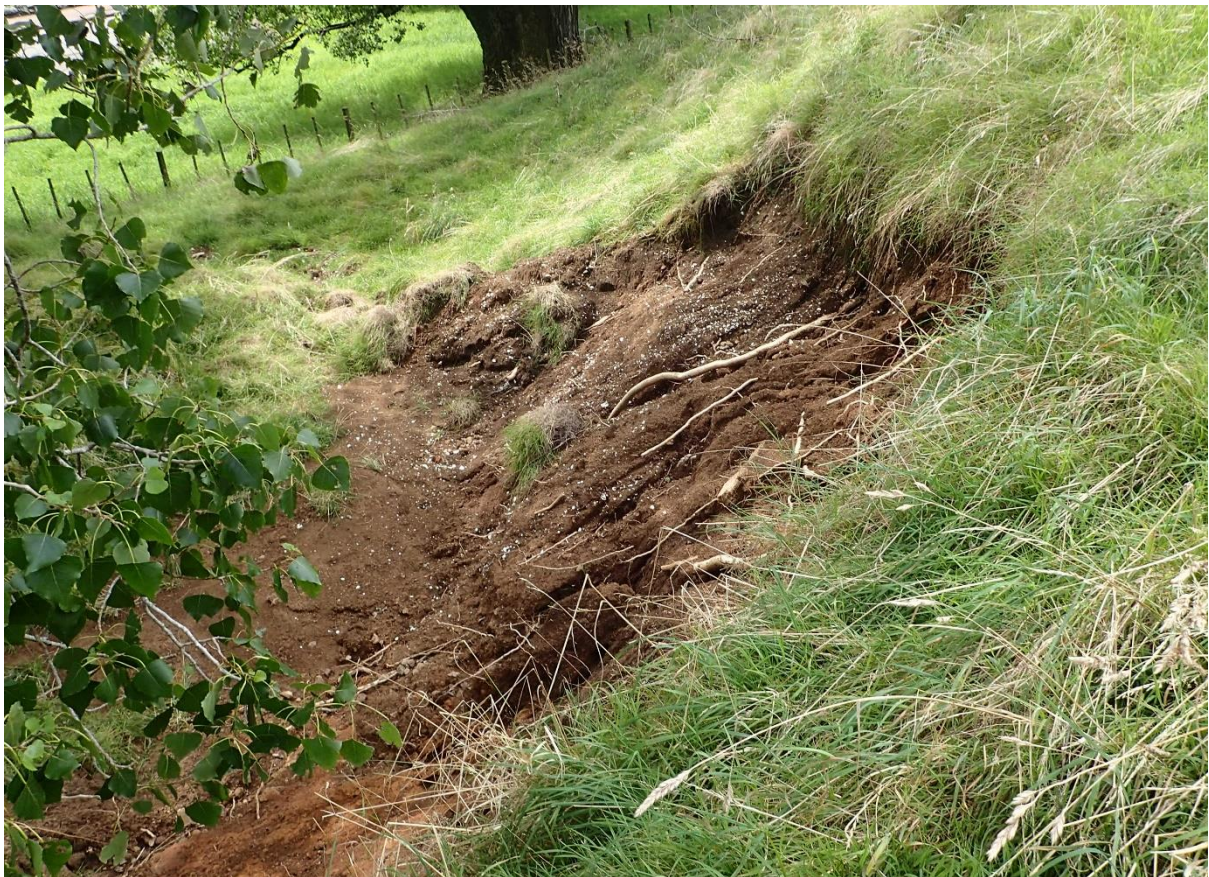
Fig. 5. Slip 9 is the only that has occurred near any tree, with some roots exposed by the slipping, which has started above and beyond the tree.
