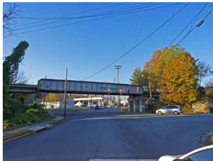
㉑ The view looking west on Northwest Blvd of the Rail Crossing and the intersection with Broad Street.
