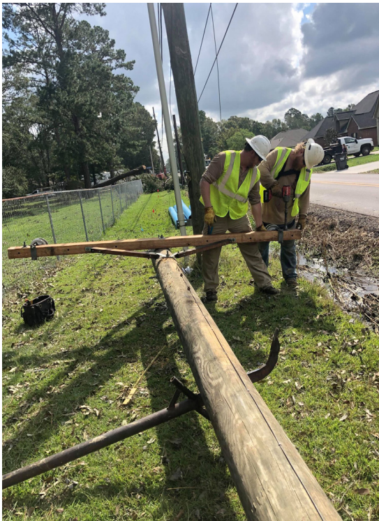
Top Right: Crews are seen working together to set one of the many new poles in the ground.
