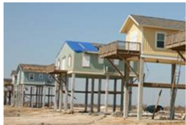
Figure 24. Wind-induced roof damage sustained by permanently statically elevated houses (image courtesy of the Journal of Light Construction)
