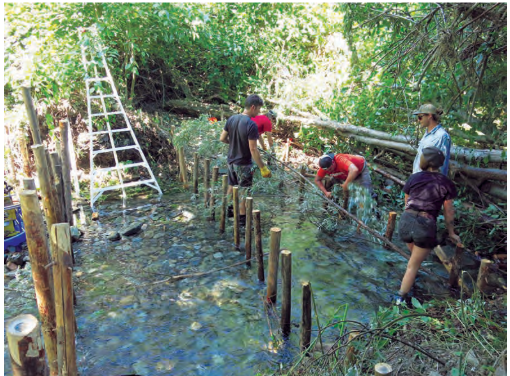
A MKWC Fisheries crew constructing BDAs. Photo by Jimmy Peterson taken August 6, 2019.
