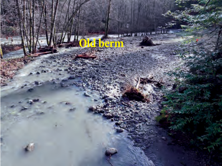
The area where the large berm used to be. The high water mark shows how the creek was allowed to expand out onto its floodplain, because the berm is gone. Photo taken January 14, 2024
