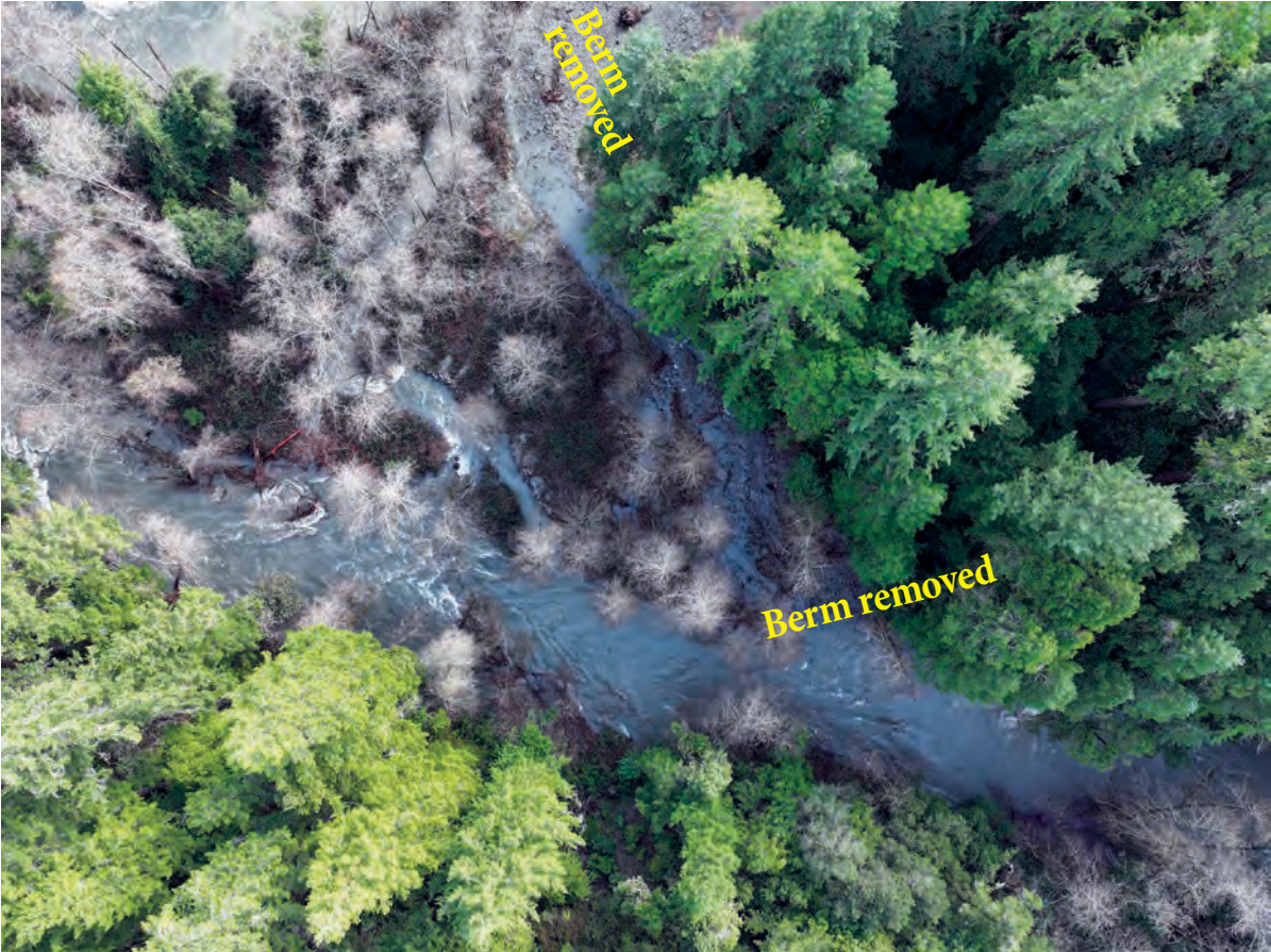
The Camp Creek restoration project site on January 14, 2024, during a large storm event (approximately five inches of rain in a 24 hour period). In 2023, MKWC, the Karuk Tribe, and Six Rivers National Forest removed two berms and old hatchery infrastructure at the site, to increase the extent and quality of spawning and rearing habitat. All photos in the Fisheries section by the MCWC Fisheries Program unless noted
