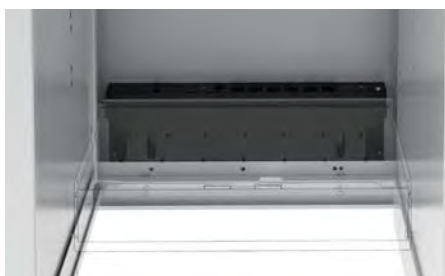
POWER FEED PANEL UNDER THE WORK SURFACE
