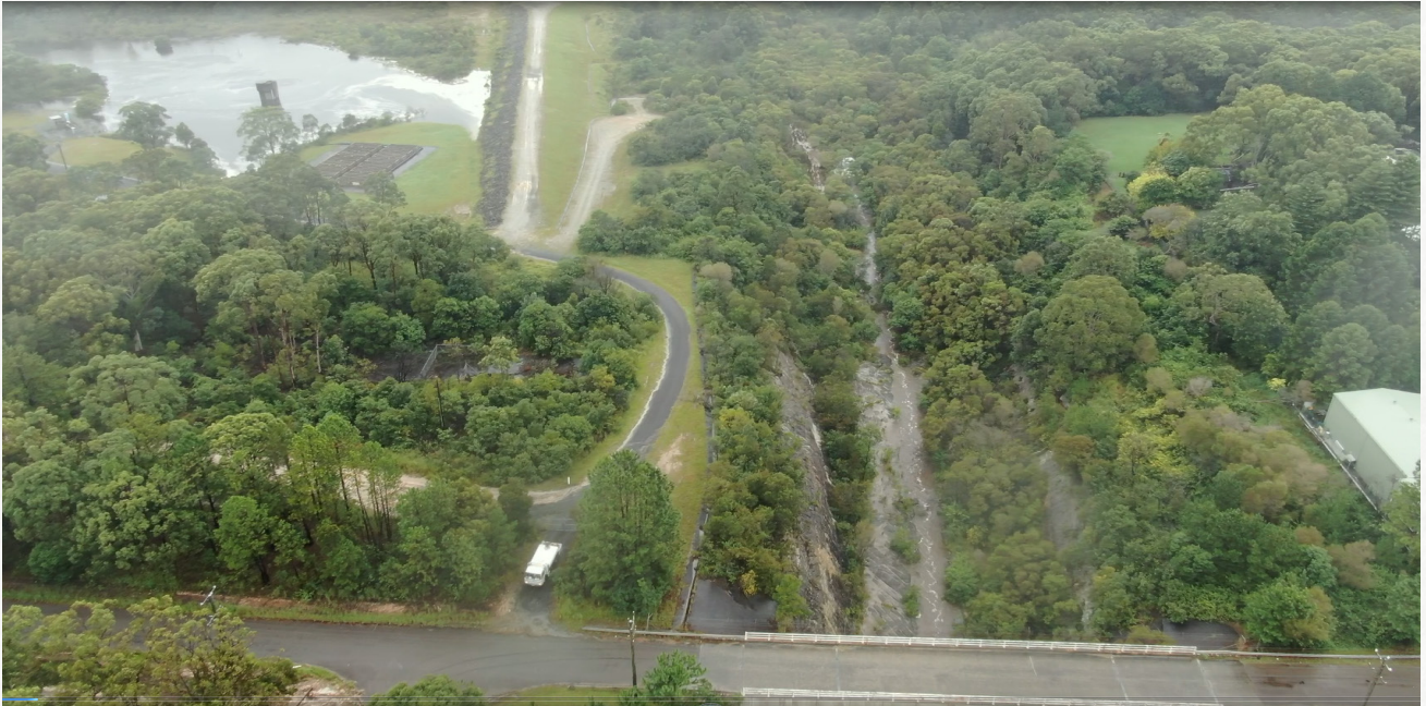
Figure 31: Current ash dam overflow at Wyee Dam wall into Wyee Creek
