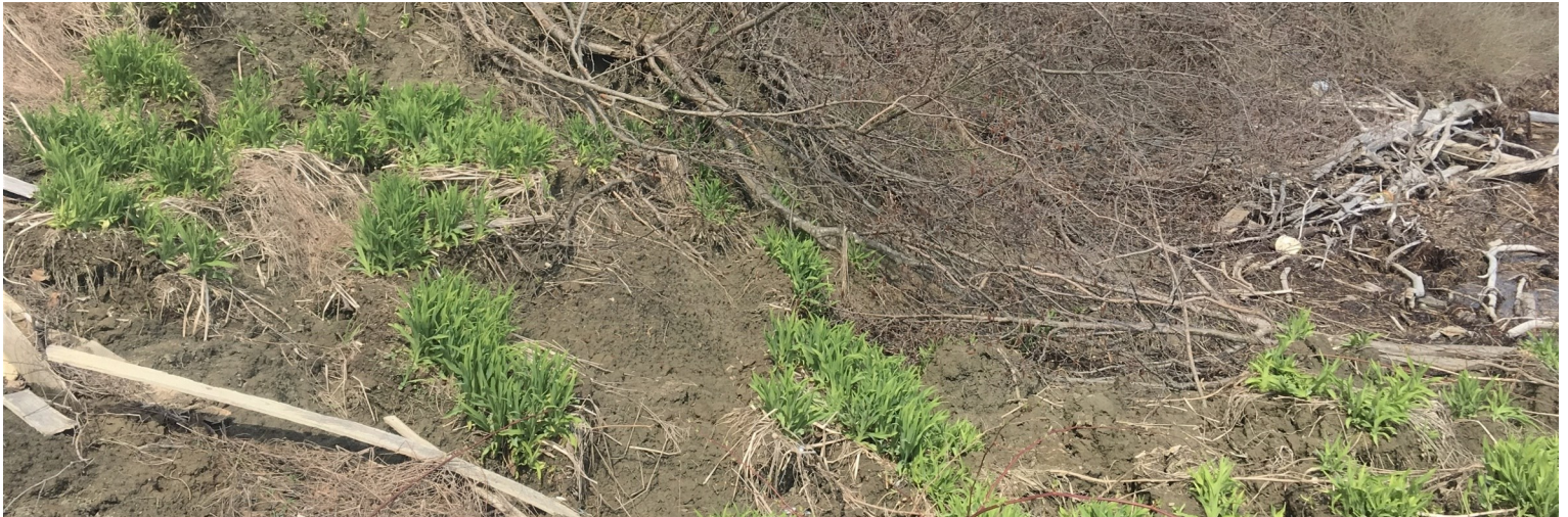
Figure 4. Plant additional woody and herbaceous planting throughout the terraces of the failure.
