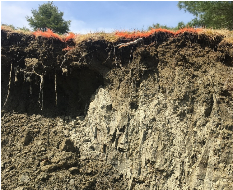
Figure 2. Clay soils visible in bluff failure at Mere Point Case Study location.
