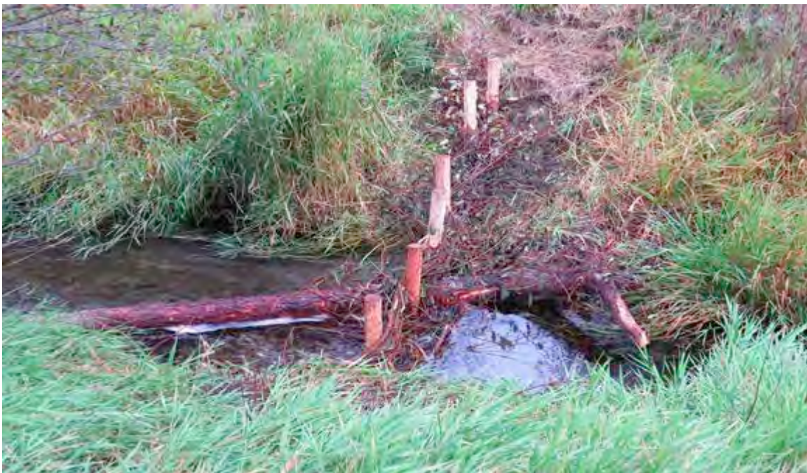
Figure 73: BDA – Two pilings extending onto the bank with LWD placed through the structure
