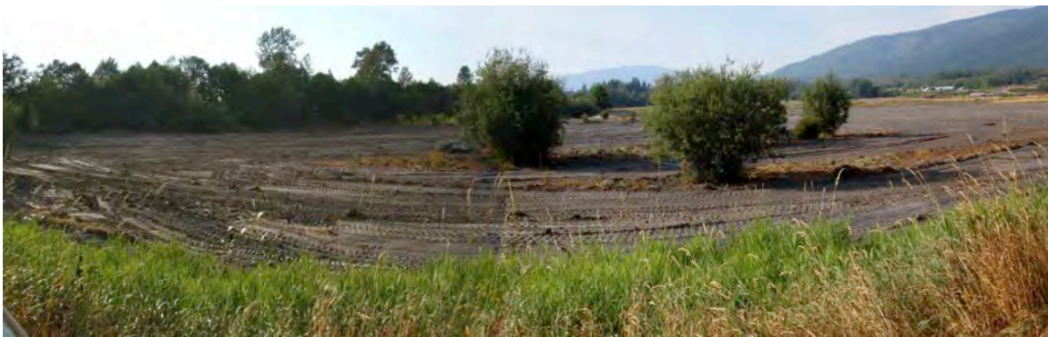
Figure 80: Photo of the restoration site during construction after removal of invasive reed canarygrass
